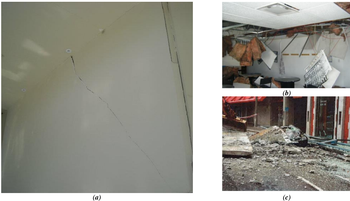
Figure 2: Component damage during the 22 nd of February 2011 Christchurch earthquake; (a) interior partitions, (b) suspended ceilings [2], and (c) precast concrete panels [17].
