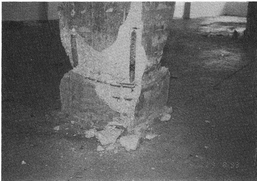
Figure 6 Inarajan High School - base of column supporting gymnasium roof
