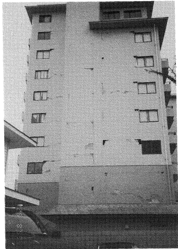
Figure 24 Damage to masonry infill panels, Royal Palm Hotel
