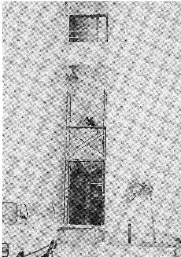
Figure 13 Severe cracking to coupling beams of Pacific Star Hotel
