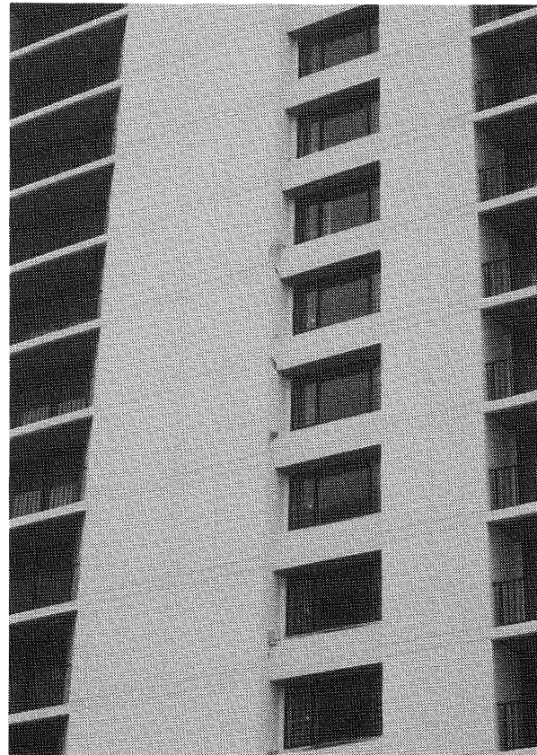
Figure 14 Minor cracking to coupling beams of the Guam Reef Hotel
