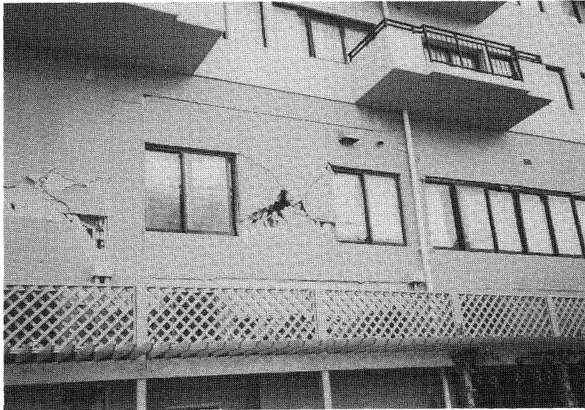
Figure 23 Damage to masonry infill panels, Royal Palm Hotel
