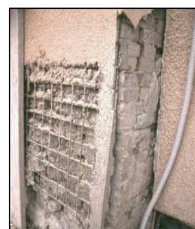
b) Loss of plaster and bond following an earthquake
