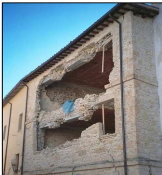
Figure 17: Eccentricity and redistribution of load in existing masonry walls due to RC beam positioning [75].
