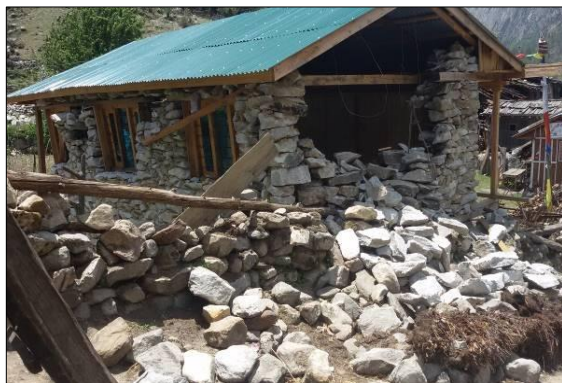
(c) Damaged dry stacked stone masonry building
