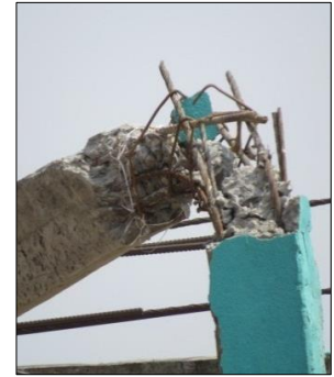
(b) Insufficient lap splice length
