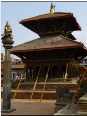
(a) Damage to smaller Pagoda temples with temporary propping to reduce further damage during aftershocks
