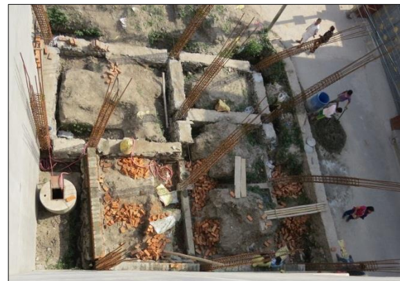
(c) Construction of foundation grid with RC ring beams and column reinforcing
