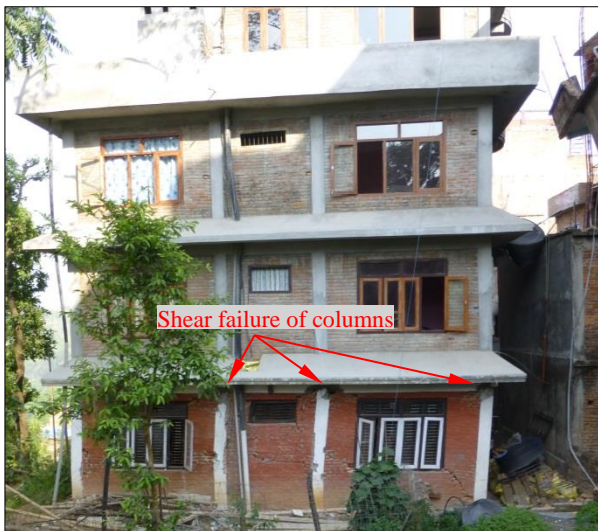
Figure 41: In-plane damage to masonry infills and significant shear failure of RC columns due to 'short-column' effect.
