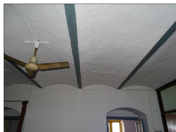
(c) Jack arched heavyweight diaphragms, with thickness ranging up to 400 mm (16") – mainly in Palace-type buildings 27°40'51.54"N 85°19'6.54"E
