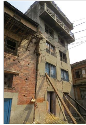
(b) Temporary propping of a near collapsing five storey residential URM building
