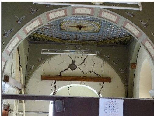
(a) Significant damage to arch
