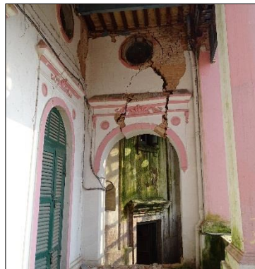
(b) Significant damage to arch
