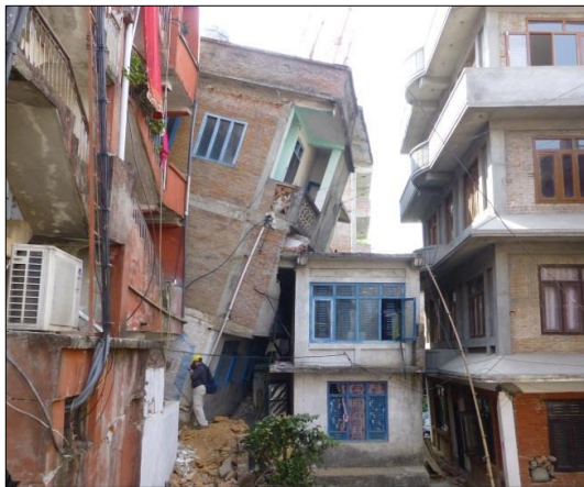
(c) Soft storey collapse example 3
