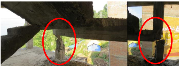
(c) Close-up of b, shear failure of columns
