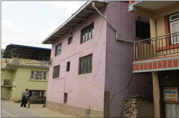
(b) Example of residential URM buildings with cement mortar and RC floor and roof diaphragms
