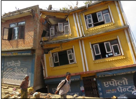
(b) Soft storey collapse example 2
