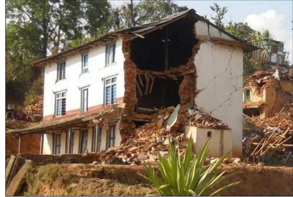
(a) Traditional stone masonry building with in-plane and corner damage
