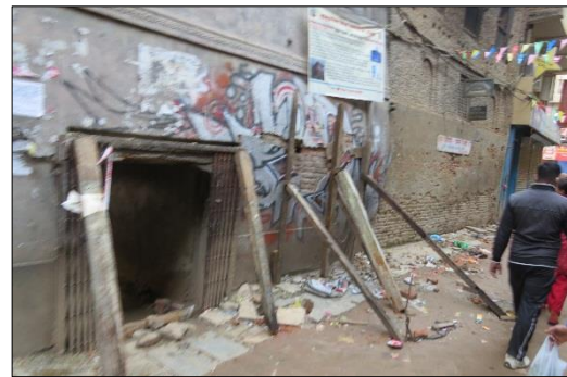
(c) Example of propping against extreme bulging of a five storey building
