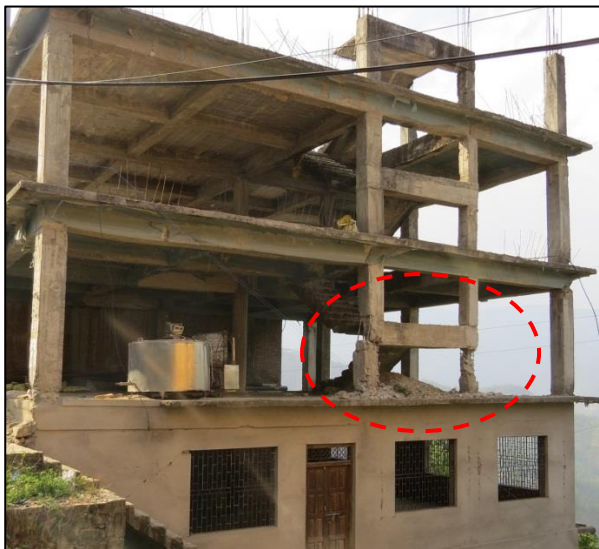
(b) Column shear failure due to stairway landing connection at column mid-height
