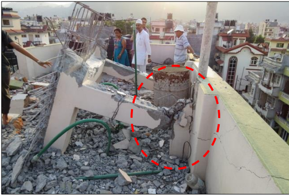
(c) Collapse of cantilevered RC support platform
