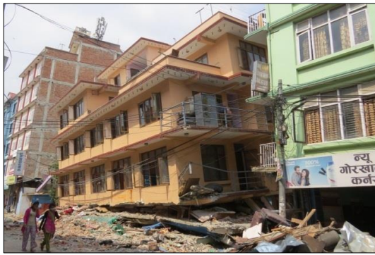
(a) Soft storey collapse example 1
