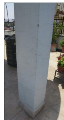
(b) Flexural cracking of cantilevered support column
