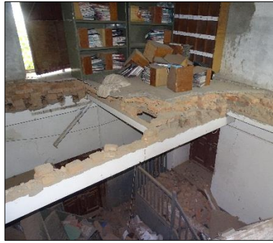
(b) Floor collapse, also showing bricks and packed mud overlying floor joists
