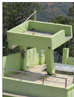
(a) Plastic hinging of cantilevered RC support columns
