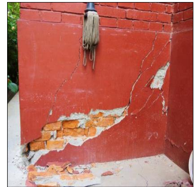
(c) Signs of toe crushing at external building corner
