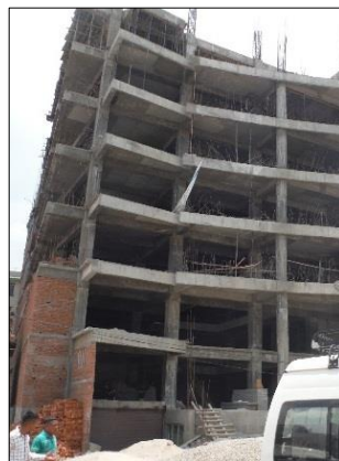
(a) Bare RC frame under construction with infills to be added later
