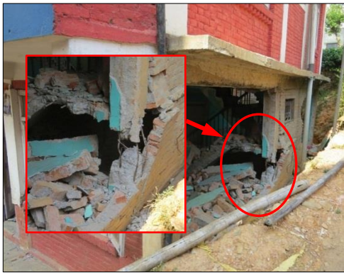
(a) Severe damage to loadbearing column in four storey building due to a staircase
