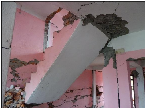
(d) Damage due to a rigid staircase
