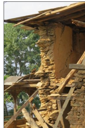
(c) Typical wall cross-section and OOP damage (Chautara)
