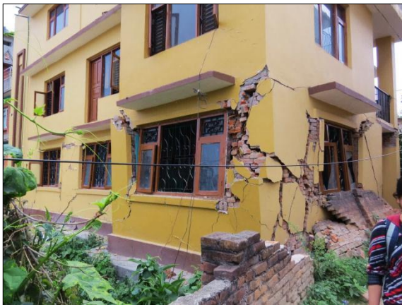
(a) Severe diagonal shear cracking of piers
