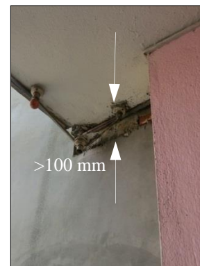
(b) Vertical differential movement due to settlement
