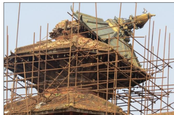
(a) Collapse of top portion of a Pagoda type temple
