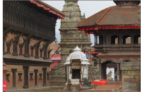
(a) Partial collapse of a small temple tower, with remaining buildings standing but with some damage
