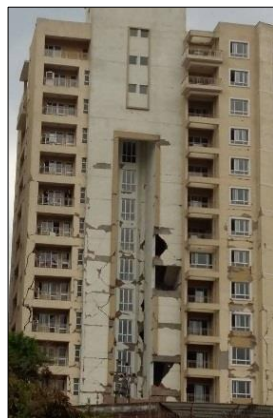
(b) Severe damage to lower floor infill walls in a multi-storey RC frame residential building
