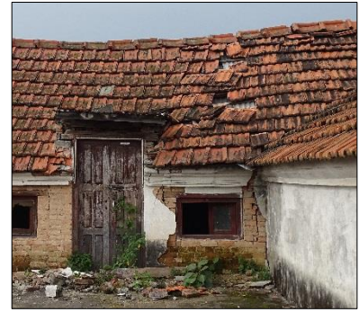
(c) Dislodged heavy roof tiles
