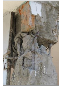
(a) Poor quality concrete
