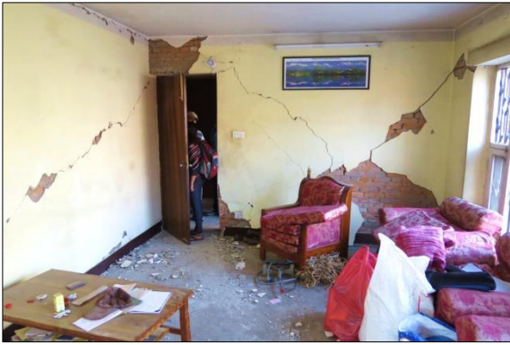
(a) Diagonal shear cracking observed in internal loadbearing walls
