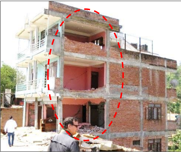
Figure 40: Out-of-plane collapse of the infill masonry walls.
