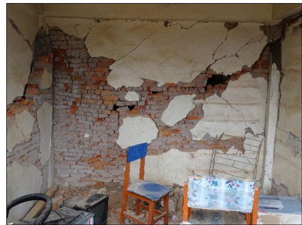
(c) Severe shear dilation of infill walls leading to failure of gravity load supporting columns
