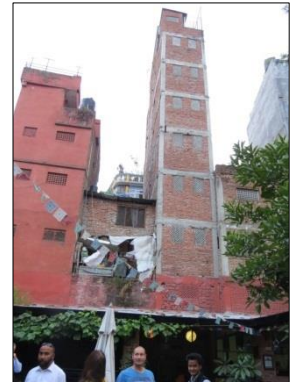
(b) Slender building with split levels and no seismic separation gaps between buildings
