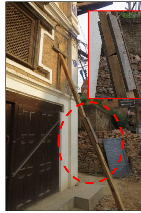
(a) Example of a splice detail with three nails per side in a timber brace
