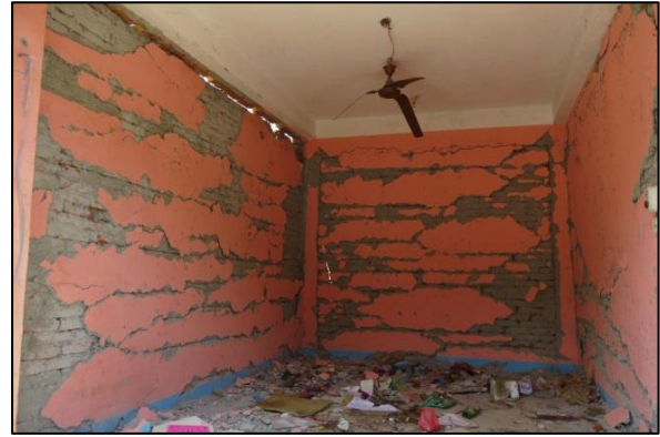
(a) Significant sliding along mortar joints and bed joint shear failures of infill masonry walls
