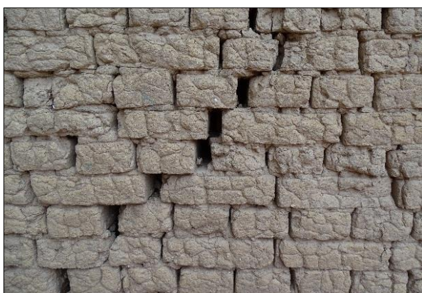
(d) Masonry construction, using English bond pattern and 'raw' clay bricks (sun dried only)
