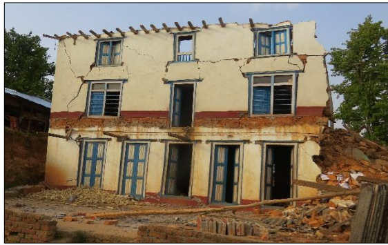
(a) Out-of-plane collapse and in-plane failures both in the piers and spandrels
