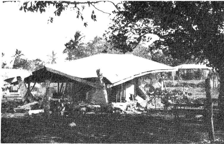
FIGURE 8: MASONRY HOUSE 'EUA - INTERNAL TIMBER PARTITIONS PREVENTED COMPLETE COLLAPSE
