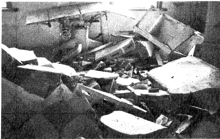
FIGURE 18: COLLAPSED UNREINFORCED MASONRY PARTITIONS 'EUA HOSPITAL
