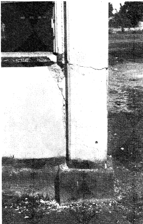
FIGURE 11: CORNER COLUMN SHOWING CRACKING AT BOTTOM AND SILL LEVEL AT TAILULU COLLEGE
