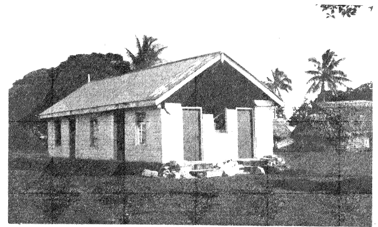
FIGURE 17: TYPICAL FAILURE OF MASONRY GABLE - NOTE TRADITIONAL FALE ON RIGHT
