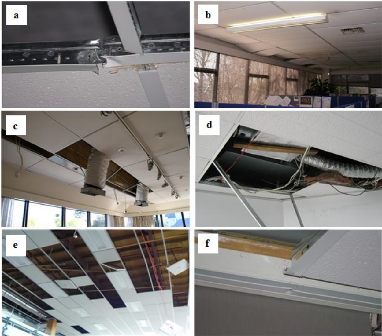
Figure 4: Failure due to (a) main tee splices; (b) perimeter fixings; (c & d) services support; (e) grid spreading; and (f) perimeter fixing damage [3].
