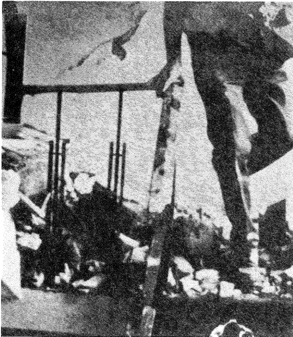
-Stairs Littered with Debris, Banco Central.
