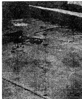
Slight ground settlement occurred around building.
