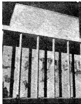
Spalled plaster off exterior of south wall.
