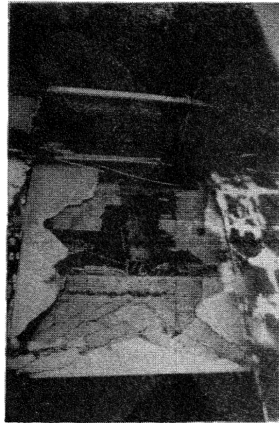
FIGURE 5b: SHEAR CRACKING IN PENT-HOUSE COUPLING GIRDER
