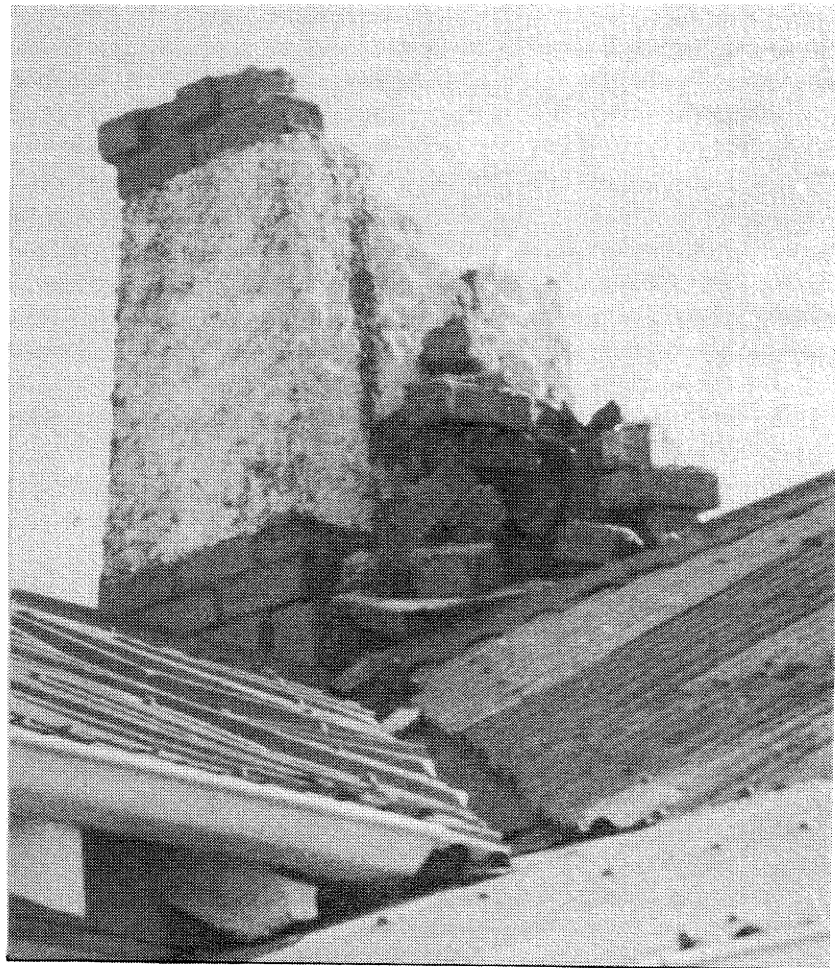
FIGURE 4: DAMAGED CHIMNEY ON HOUSE IN BAYVIEW ROAD, ST KILDA. NOTE THE COMPLETE SEPARATION OF THE COMPONENT BRICKS. PHOTOGRAPH LOOKING SOUTH-EAST.
