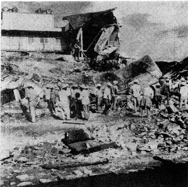
FIGURE 8: THE "PACKARD" APARTMENT BUILDING, WORKMEN ARE STANDING ON WHAT WAS THE REINFORCED CONCRETE ROOF OF THE THREE-STORY COMPLEX.
