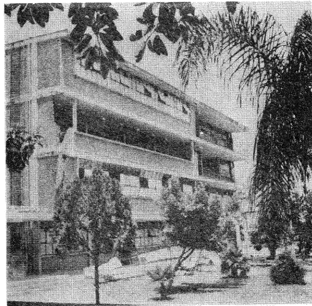
FIGURE 13: DAMAGE TO BUILDING B, TECNOLOGICO OF ORIZABA.
