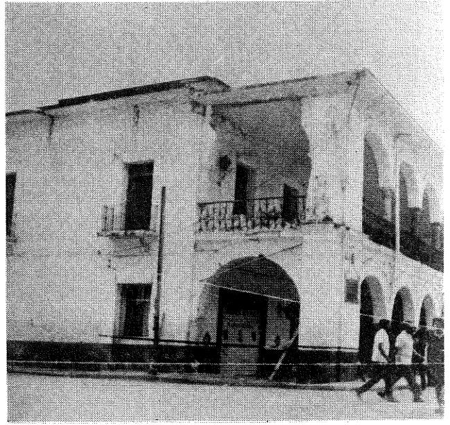
FIGURE 21: DAMAGE TO EXTERIOR CORNER OF THE HOTEL ZEVALLOS, CORDOBA.
