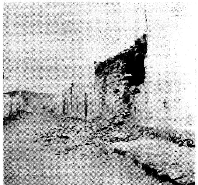
FIGURE 25: TYPICAL VIEW OF DAMAGE TO HOUSING IN SERDAN.
