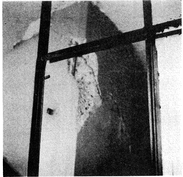
FIGURE 15: TORSIONAL CRACKING OF SECOND-STOREY COLUMN, BUILDING B, TECHNOLOGICO OF ORIZABA.
