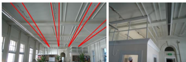
Figure 22: Underside of flooring system with location of cracking indicated by bold lines.
