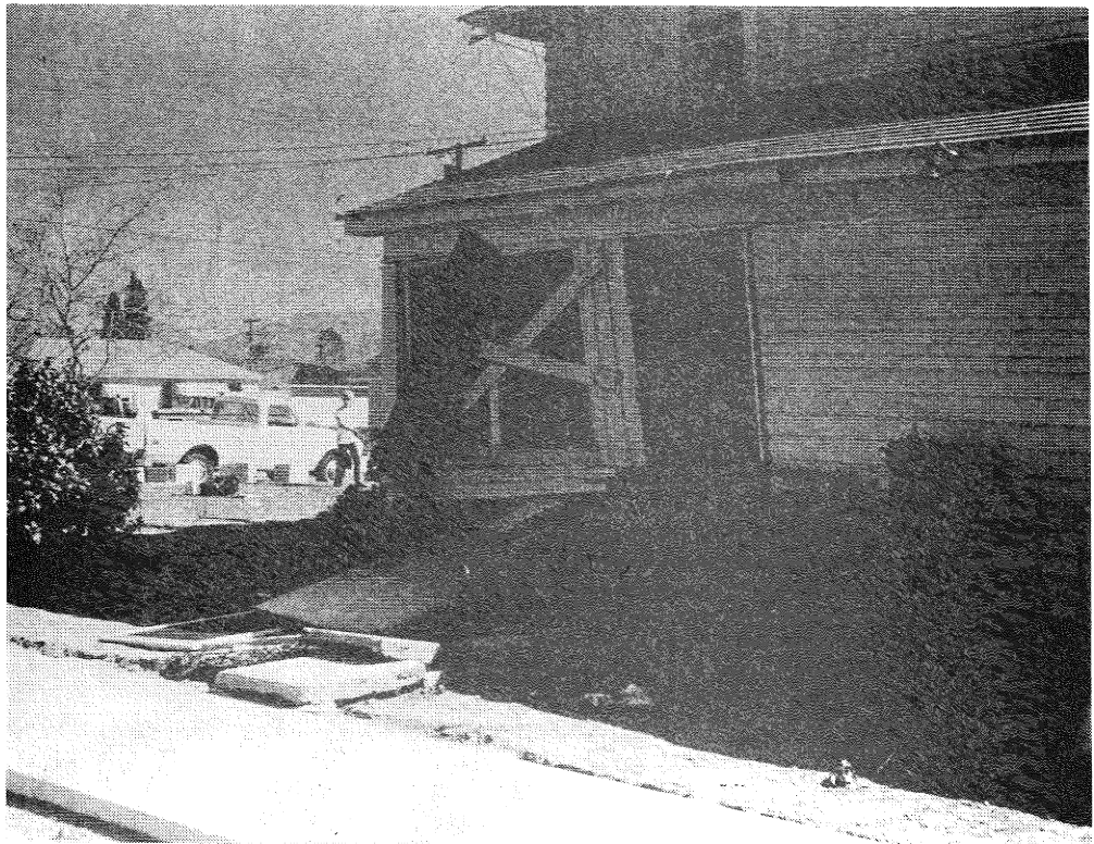
Fig 8. House in Orange Grove Avenue, thrown off foundation towards camera. Note door step forced upwards.
