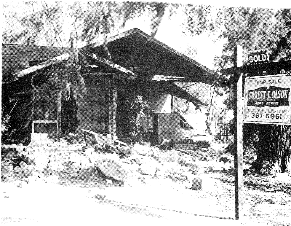
Fig 9. Collapse of brick walls of house in Eighth Street.
