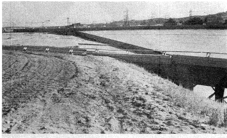
Fig. 25 Backfilling settlement and pavement failure at the eastern abutment of the Northbound Truck Route Undercrossing. Note the separation of the pavement from the abutment recess resulting in a potential barrier for emergency vehicles.
