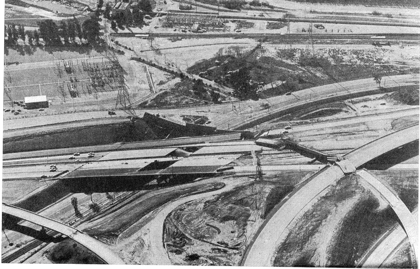
Fig. 12 The Golden State - Foothill freeway interchange, looking west. This view was taken several hours after the earthquake. The San Fernando Road transition bridge, lower left, was still intact at this stage but note the vertical sag produced by a failure at the column base.
