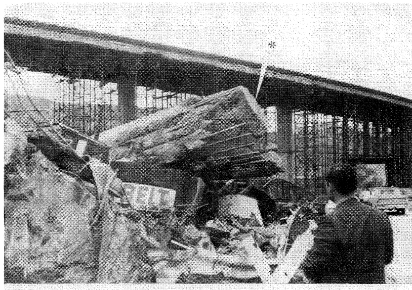
Fig. 7 Top of the collapsed column of the South Connector Overcrossing. Apparently the deck was cast on top of the flat surface at the column end.* Remains of the capping beam were not visible and must have stripped from the column during failure.
