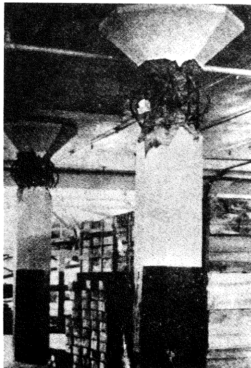
Fig. 6.19 Example of a Failed Column Hinge.
