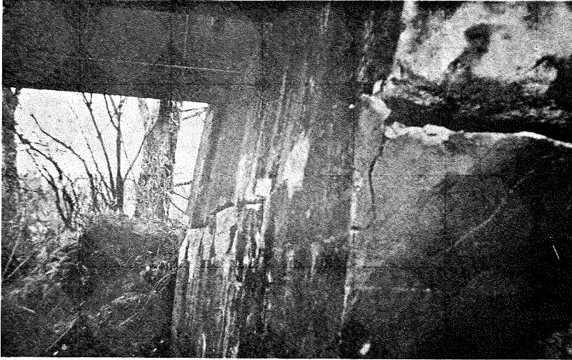
Fig. 2 Reefton buttress of the Inangahua road-rail bridge, looking upstream. Soil has thrust the buttress towards the river, causing the fracture shown.
