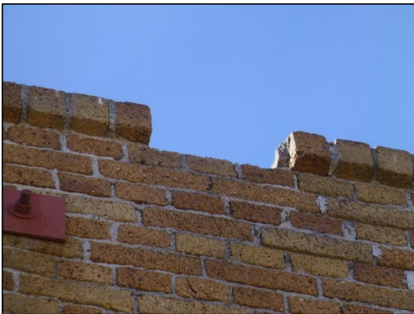
(c) Loss of capping bricks to a building in Vallejo
