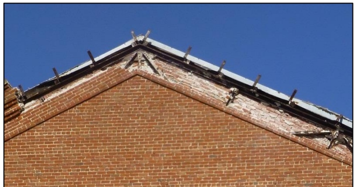
(b) Parapet failure at Mare Island
