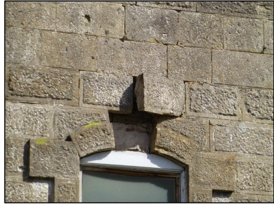
(b) Loose stones above window opening
