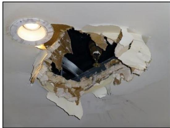
(b) Water sprinkler that was activated during earthquake
