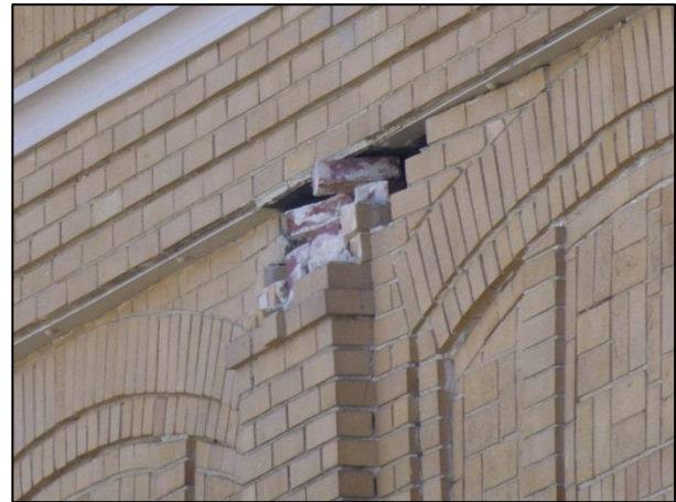
(d) Loss of brickwork above one pier, resulting in a falling hazard
