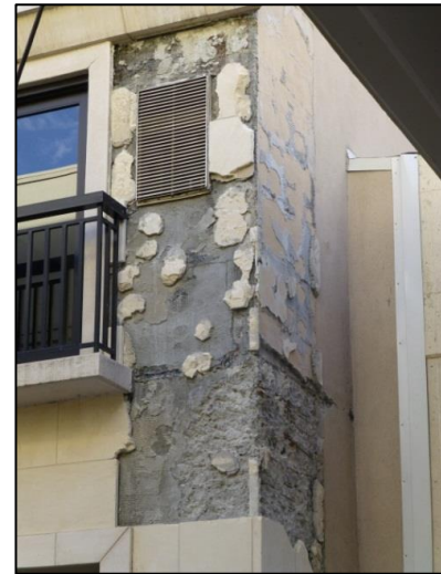
(b) Loss of exterior cladding
