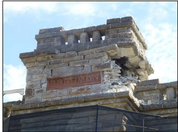
(b) Damage to the ornamental feature atop the Goodman Library in Napa
