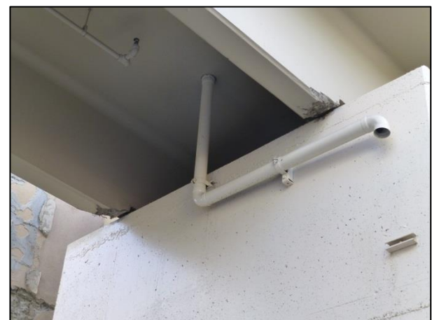
(b) Pounding damage for a pedestrian overpass
