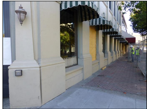
(d) Cracking at base of piers, suggesting pier rocking
