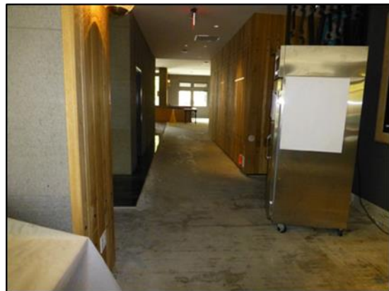
(d) Removed floor linings due to water damage
