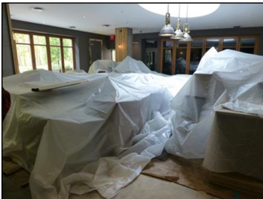
(c) Hotel furnishing covered while non-structural damage was attended to
