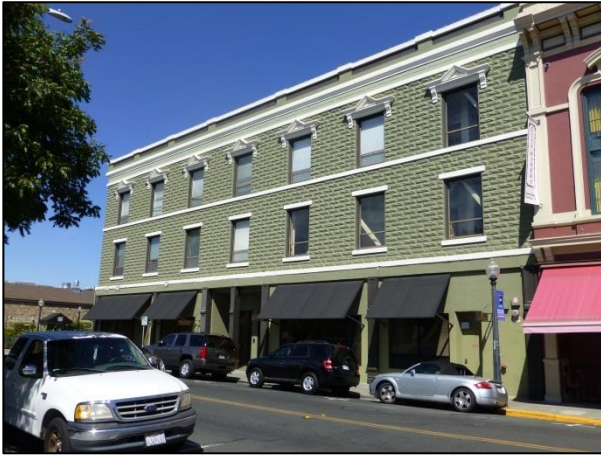
(a) Street view of building, with diagonal bracing visible in some windows
