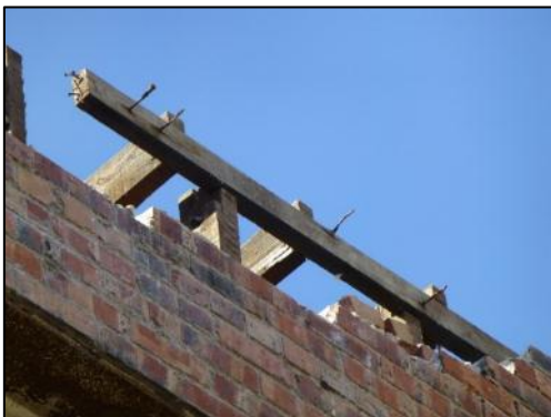
(a) Parapet failure in Vallejo
