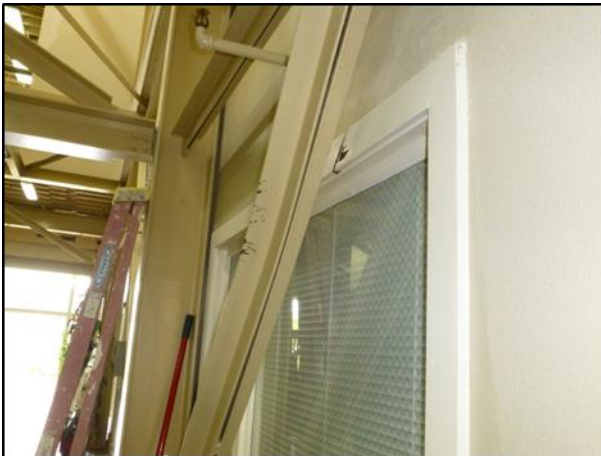
(e) Evidence that brace had buckled and come into contact with window frame
