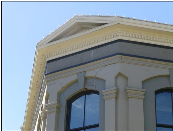
(c) Spandrel failure wrapping around corner of building
