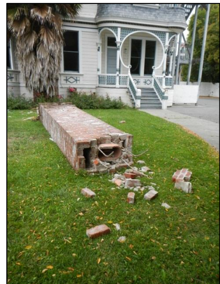
(d) Chimney completely removed (CA EQ Clearinghouse / Source: David McCormick)
