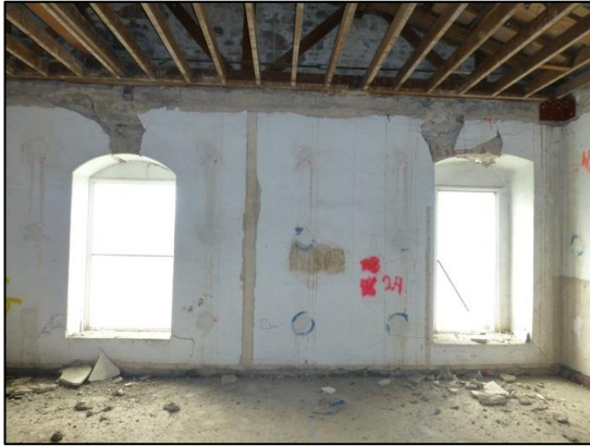
(c) Internal spandrel damage
