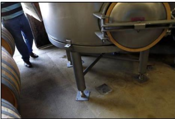
(a) Sliding of steel tanks [63]
