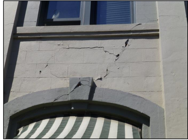
(b) Close-up view of distinct spandrel failure
