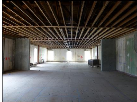
(d) Supplementary concrete walls to provide added strength and stiffness in the transverse direction
