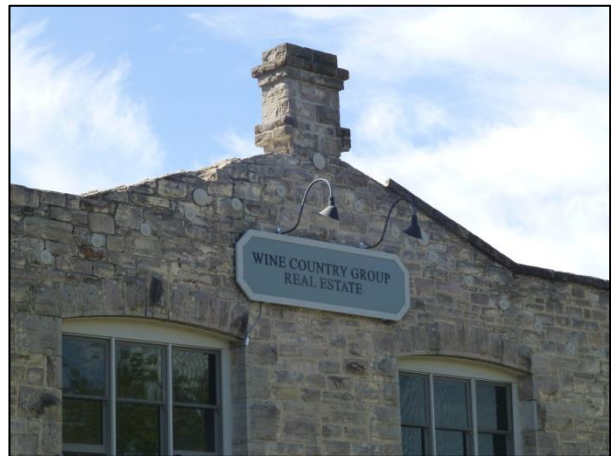
(d) Loss of capping stones to a stone masonry building in Napa
