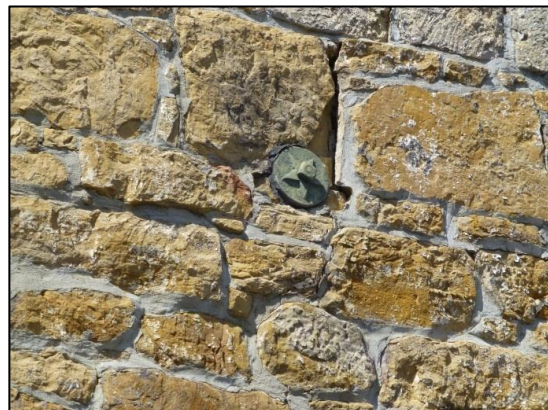
(f) Distressed stonework around the anchor plate of side-wall anchorage
