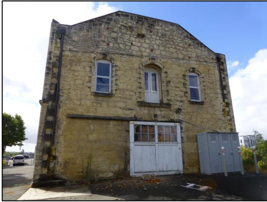
(a) Isolated fallen stone on building exterior
