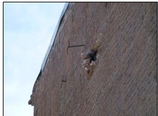
(a) Apparent rupture of the anchor rod or failure at the diaphragm connection
