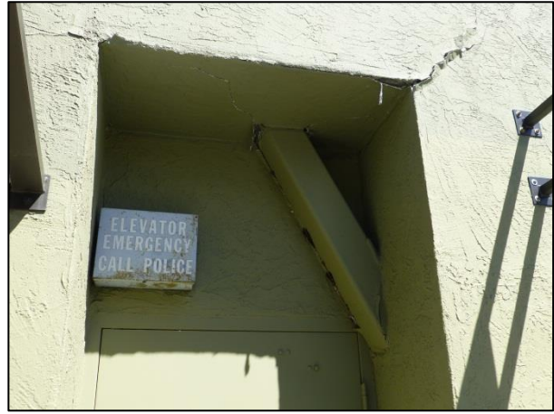
(b) Evidence of building deformation visible in recess on building exterior
