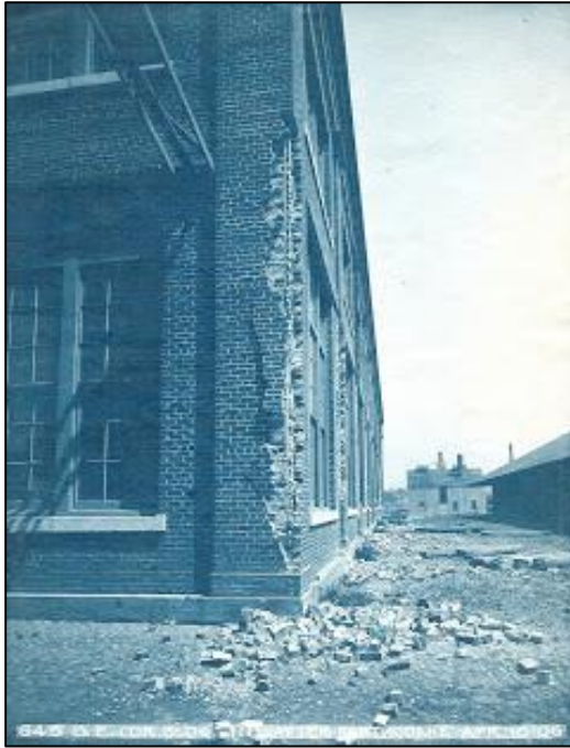
(a) Damage at Mare Island [13]
