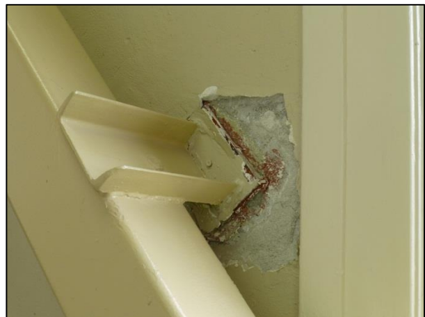
(f) Distress at connection between steel framing and URM exterior wall
