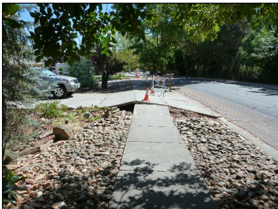
Figure 7: Buckling of pavement on Patrick Road, Napa.
