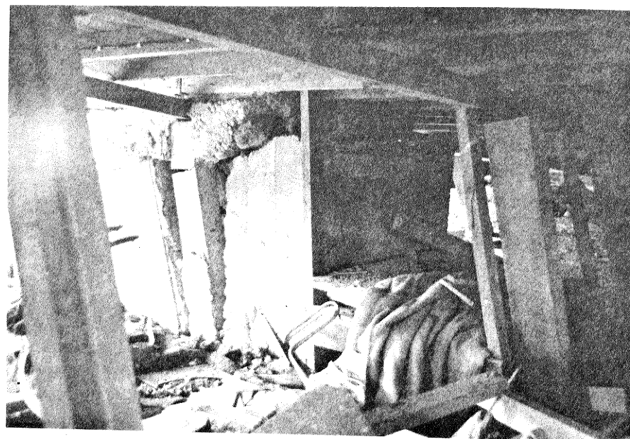
Fig. 31. Damage to chimney base fig. 25
