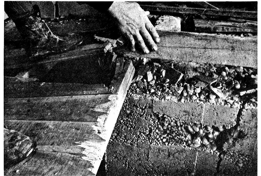
Fig. 20. Detail of fig. 19, flooring lifted on chimney base
