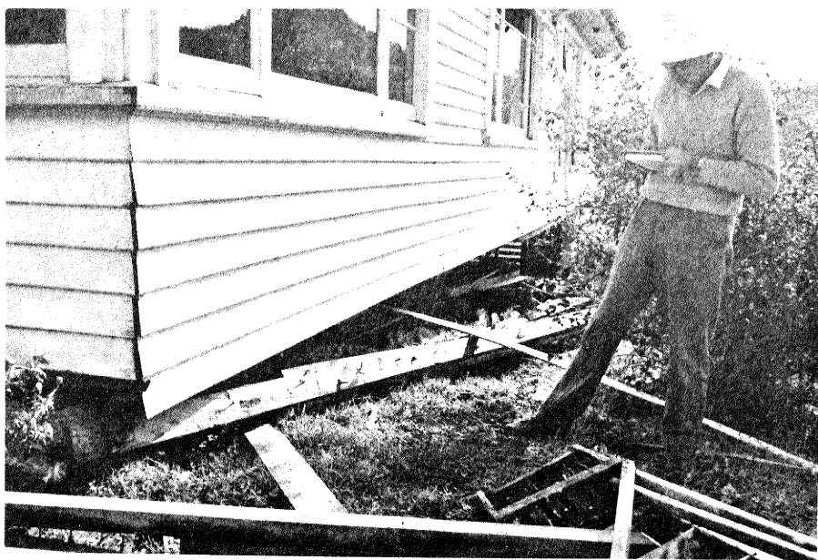
Fig. 29. Survey being made of damage and plan for repair
