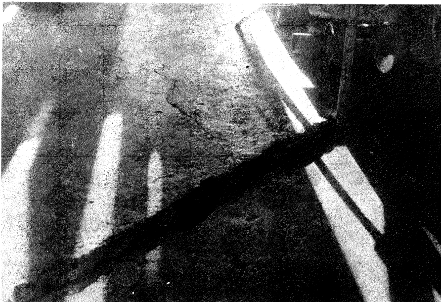
Fig. 7. Motor garage building in Reefton. Differential movement of floor slab at construction joint, in shw
