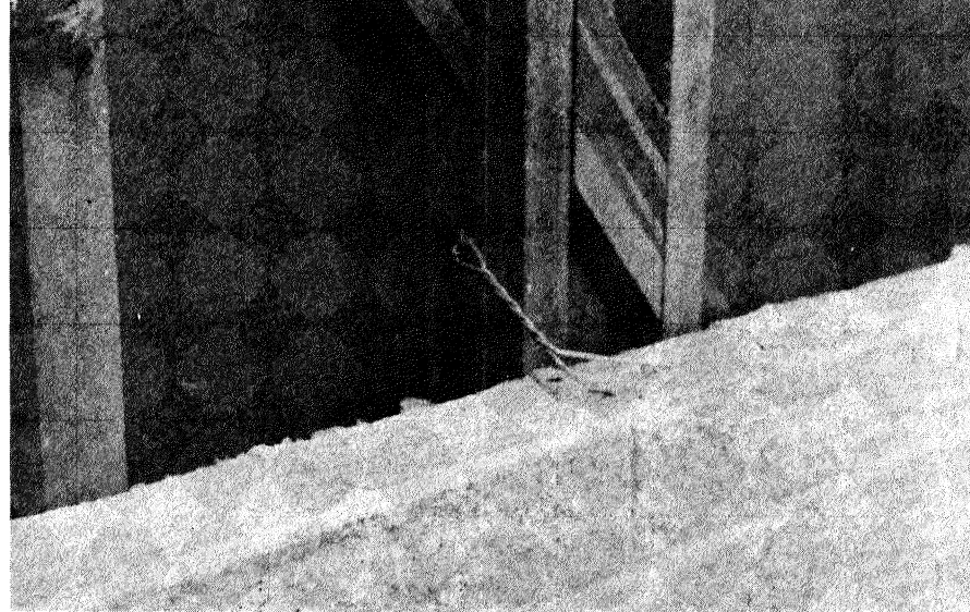
Fig. 6. Motel in Reefton. Staples of 14 gauge pulled out allowing blockwork veneer to separate from the structure
