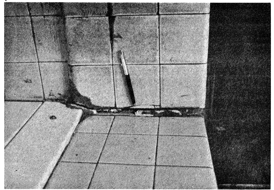
Fig. 3. Old movement & prior evident repair at fire surround
