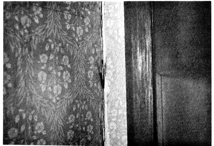
Fig. 4. Old movement and prior filling at wall junction
