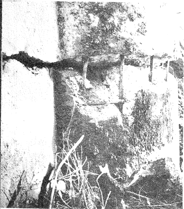
Photo 10.3: Pier 2 failure at ground level, northern face, west side. Note size of crack.
