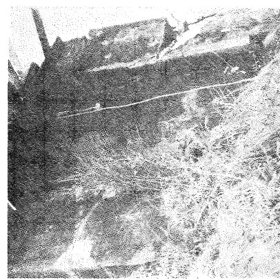
2.2 Damage at Pier 1 due to longitudinal movement.
