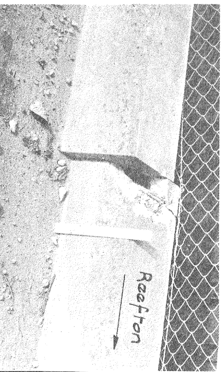
Photo 14.5 : Road deck, east side, over pier 8, showing evidence of violent longitudinal motion. West
