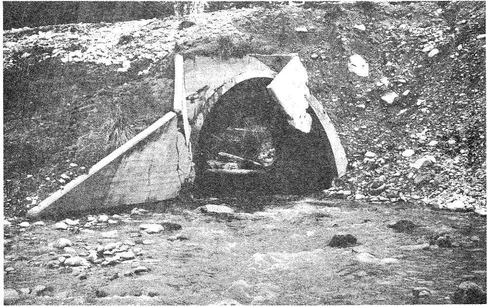
S.H.G R.M. 182.55 De Filippi Culvert damage
