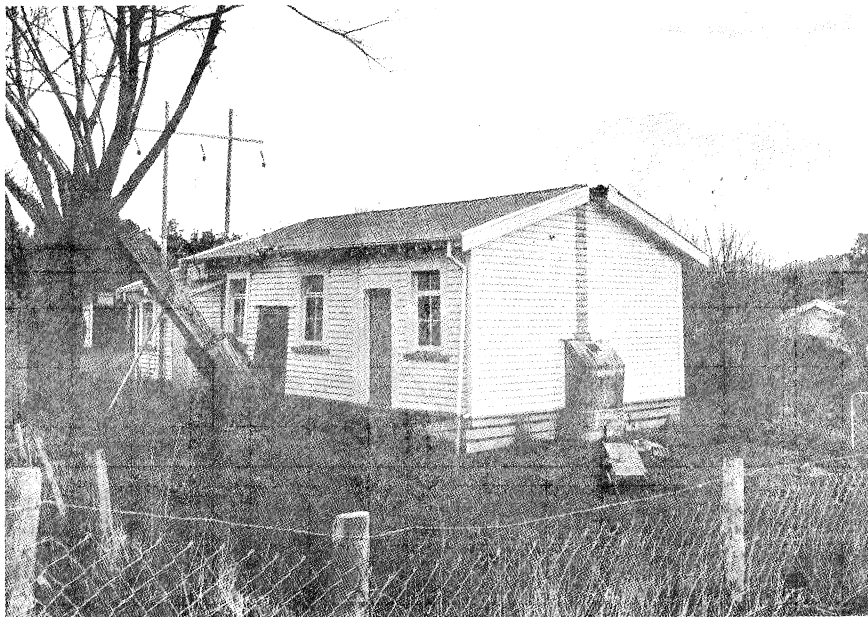
Fig. 18. Dwelling, one chimney folded out, another collapsed
