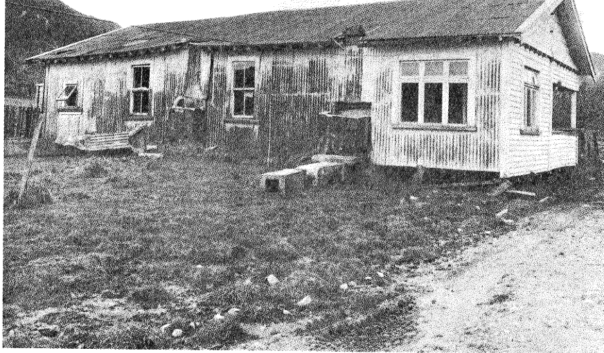
Fig. 5. Dwelling, off piles, chimneys down, 3 km n.w. of Lyell
