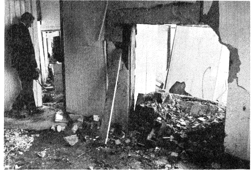
Fig. 23. Collapsed chimney and fireplace, fig. 21
