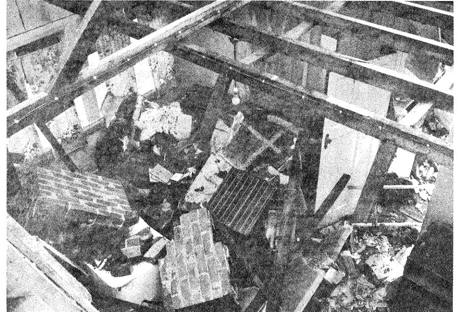
Fig. 16. Debris of tiles and chimney on living room furniture
