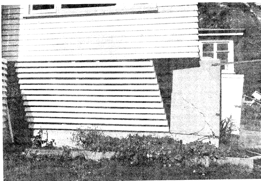
Fig. 30. Dwelling of fig. 29. movement at foundations
