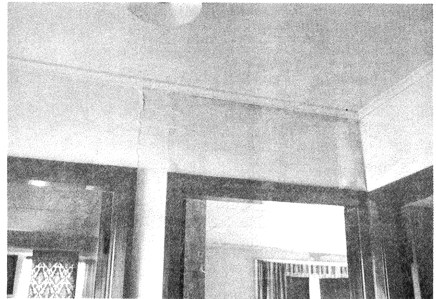
Fig. 12. Interior of fig. 10, moderate damage to lining
