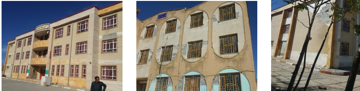
Figure 7: Damage caused by the earthquake in schools with brick facades.
