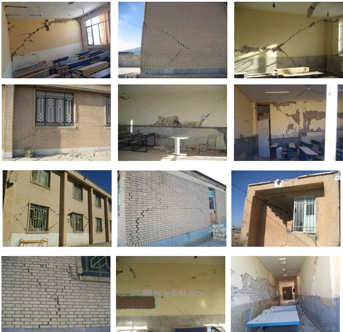
Figure 9: Damage sustained by unconfined schools located within 10 km radius of the epicentre.
