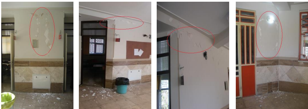
Figure 14: Surface cracks on the anchored infill walls of schools 10 to 40 km away from the epicenter.
