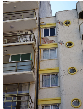
(b) Tilting of the left building leading to pounding.
