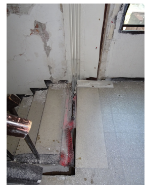
(b) Stairs failure (side view).
