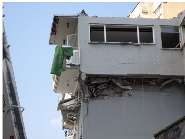
(c) Storey collapse of level 5.
