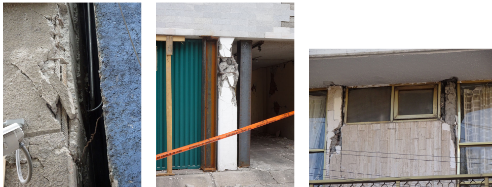
(e) Lap-splice with insufficient length and confinement leading to debonding of concrete.
