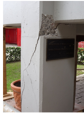
(a) Shear crack in a column of administration building.
