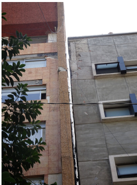
(a) Damage due to pounding between two buildings.
