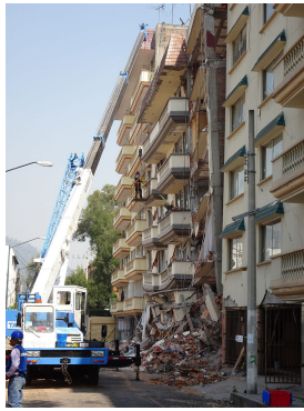
Figure 12: Soft storey failure leading to building collapse.
