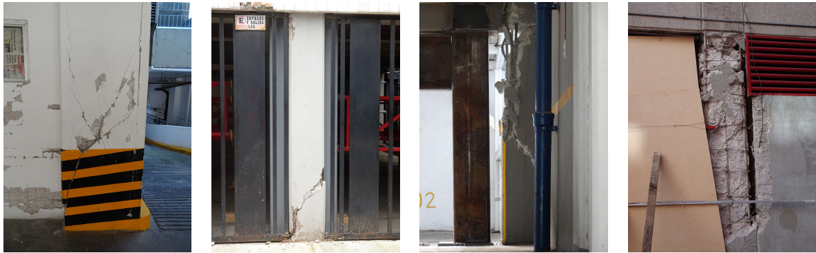
(a) Shear failure in a column.
