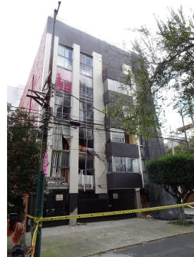
(b) Damage on the North facade.
