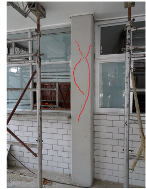
(b) Shear crack in a column of administration building.
