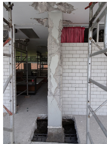
(c) Damage to a column in the Kindergarten.
