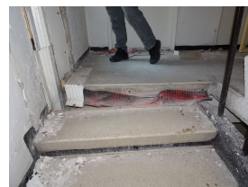
(a) Stairs failure (front view).
