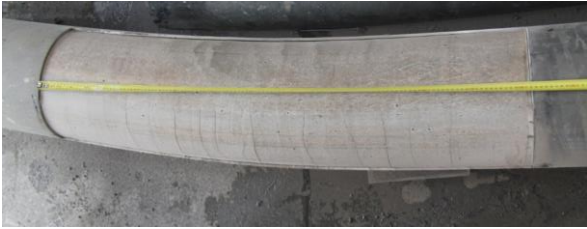
Figure 20: Post-test examination of BRB 6.5 showing cracking underneath steel casing.
