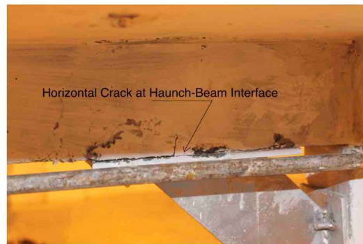
Horizontal Crack at Haunch-Beam Interface
