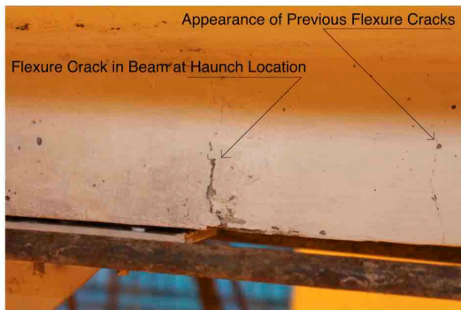
Slight Flexure Cracks in Beam on Ground Floor
