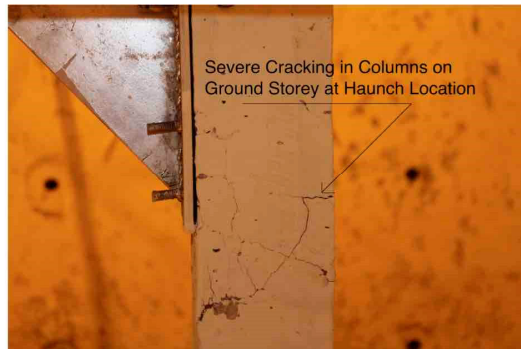
Severe Cracking in Columns at Haunch Location
