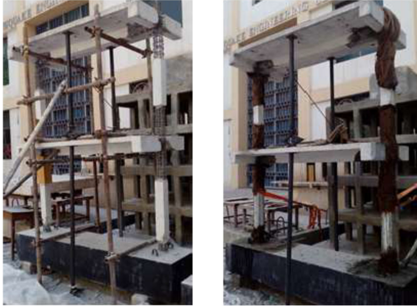
Figure 4: Replacement of damaged concrete: (left) Damaged concrete removed at the connection; and (right) New high-strength concrete was used as a replacement.
