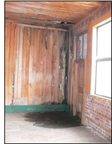
(b) Evidence of decay due to moisture.
