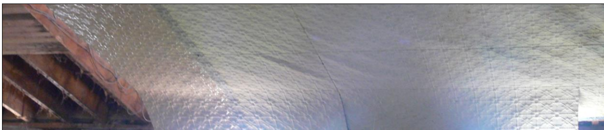
Figure 14: Patterned 0.3 mm tin ceiling lining underlying a straight sheathed flexible timber ceiling diaphragm.
