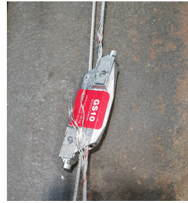
(a) Damage near the grips.
