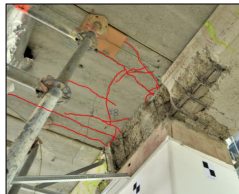
Figure 2: Soffit damage in a ‘beta unit’ recorded following the 2016 Kaikōura earthquake [29].
