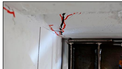
(d) Vertical offset in soffit crack of beta unit U5 (North support) at -1.84\% ( \parallel ) drift.
