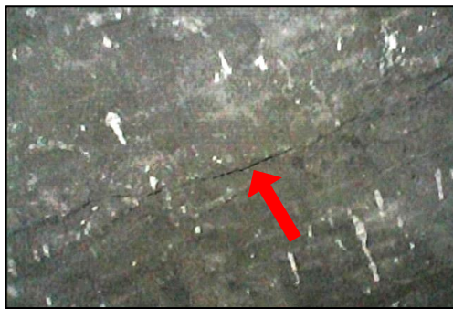
(a) First web crack at the south end of unit U8 at -0.42\% ( \parallel ) drift.
