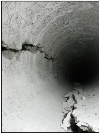
(a) Internal damage recorded at 2% drift [8].
