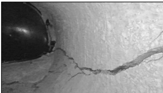
(a) Web cracking at the north end of unit U8 at -2.42% (||) drift.
