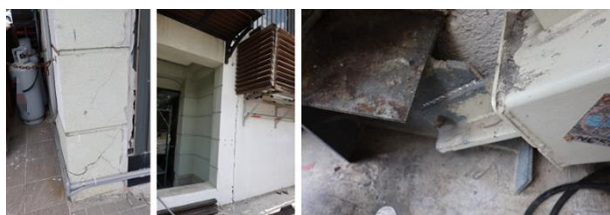
Figure 12: Observed damage to Building A11.
