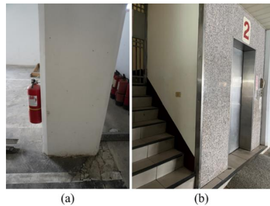
Figure 8: (a) manual fire extinguishers and (b) functional elevator post-earthquake in Building S03.
