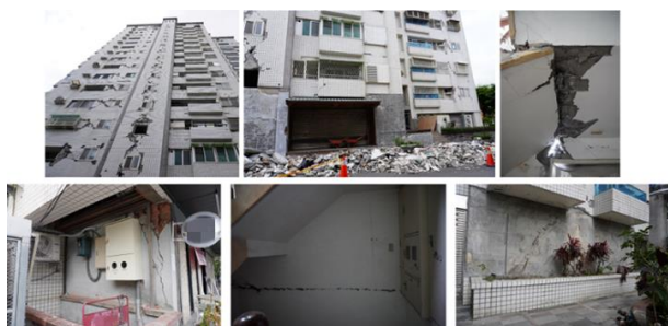
Figure 14: Observed damage to Building D13.
