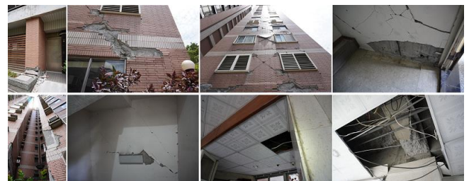
Figure 20: Observed damage to Building O67.
