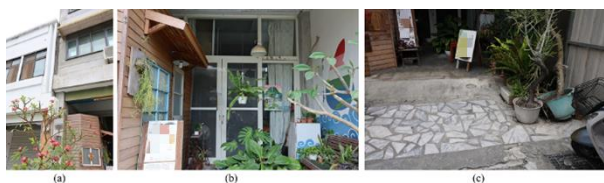
Figure 18: (a) pounding damage to the adjacent building, (b) door jamming, and (c) pavement cracks and content damage.
