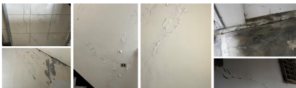
Figure 7: Observed damage to Building S03.
