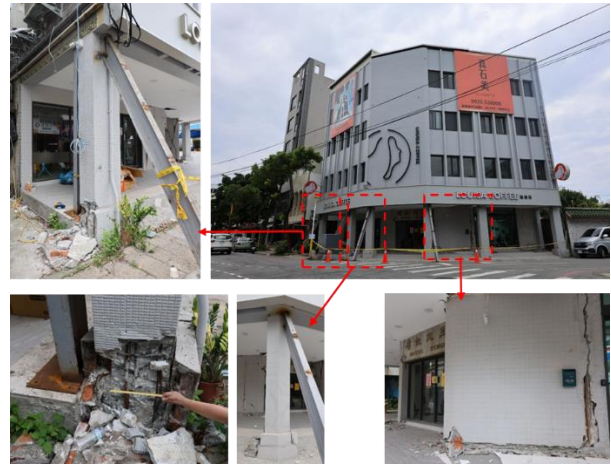
Figure 26: Damaged Building – shoring added after mainshock.
