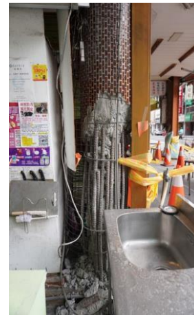
Figure 21: Lap-splices and lack of confinement and concrete cover at the base of column.
