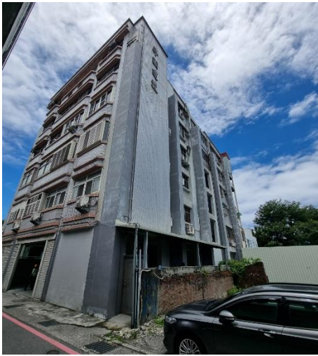
Figure 30: Retrofitted building – strengthened after the 2018 Hualien Earthquake, with no observed damage following the 2024 Hualien Earthquake.
