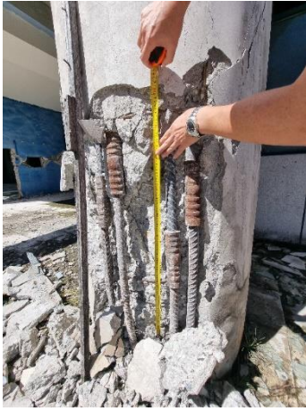
Figure 23: Longitudinal reinforcement bars spliced using mechanical couplers cast outside the spiral used as transverse reinforcement.
