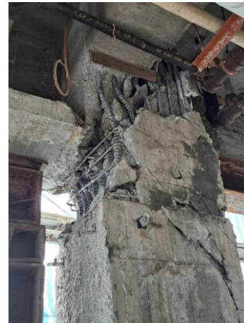
Figure 22: Lack of shear reinforcement in column and beam column joint.
