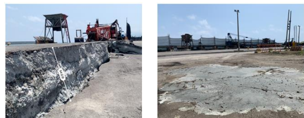
Figure 19: Damage to the port. a) Some of the port areas uplifted up to 50 cm. b) Sand boils and surficial signs of liquefaction.
