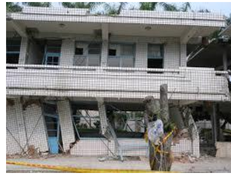
Figure 29: School building damaged in the 1999 Chi-Chi Earthquake) [29].
