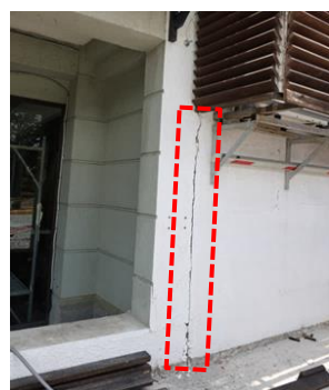
Figure 31: Cracking at seismic joint between Buildings A11-1, A11-2.
