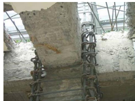
(c) Beam-column joint with RC column jacketing. Figure is taken from Chiou [3].
