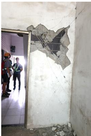
Figure 28: Shear failure in RC shear wall of Building C05.
