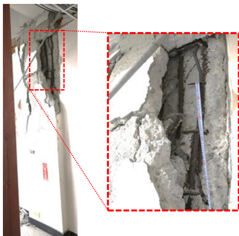
Figure 41: Axial failure of column consisting of buckling of longitudinal reinforcing bars in Building E35.
