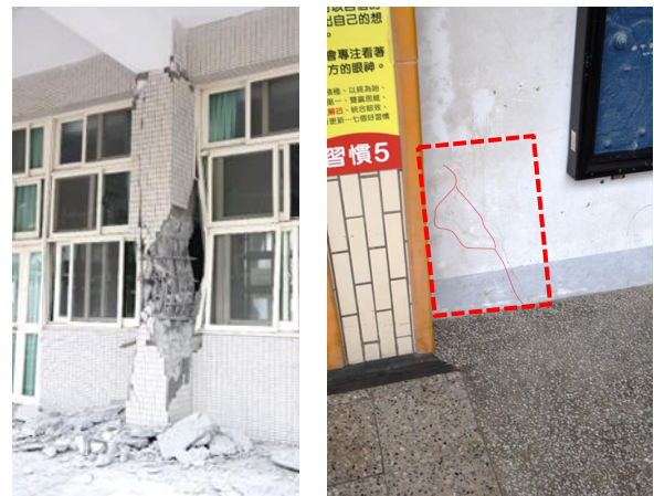
Figure 20: Shear and axial failure of typical column in Building S01. (Source: Shegay [10])
