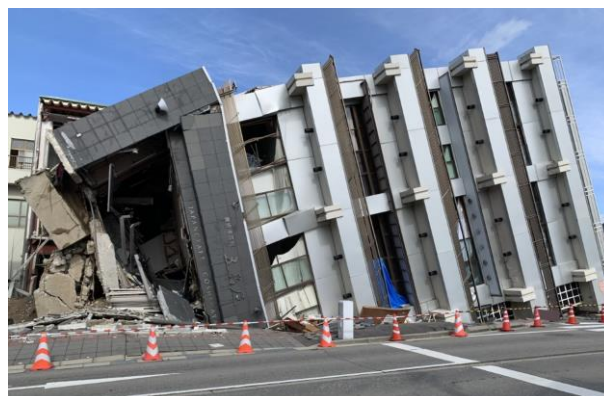
Figure 5: Pile cap failure in a 5-storey apartment building in Wajima.
