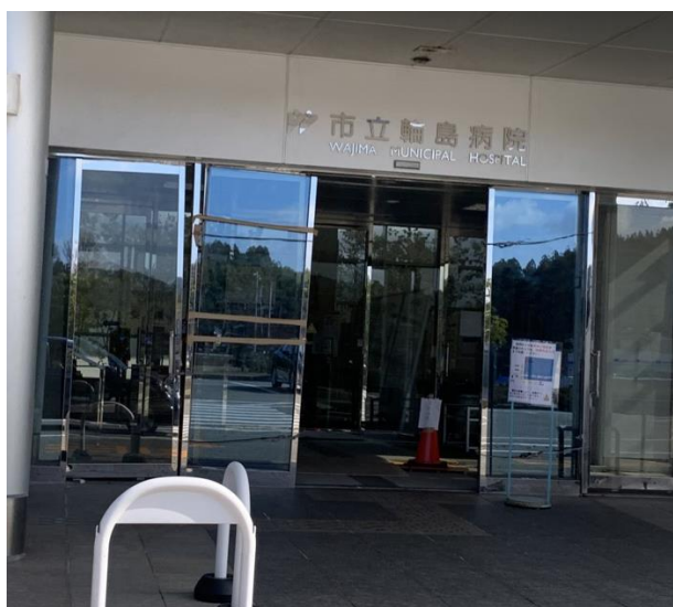
Figure 4: Non-structural damage to the hospital doors causing them to be strapped open in sub-zero temperatures. A great example of the need for displacement capacity in critical non-structural elements.
