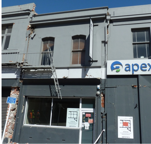
Figure 1: Pounding damage observed in the 2011 Christchurch earthquake.
