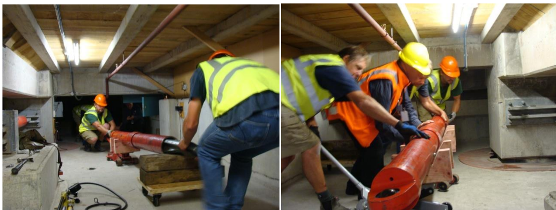
Figure 12: Left, damper being transferred to trolley. Right, damper returned to floor jacks ready to be lifted to correct height and rolled into position.
