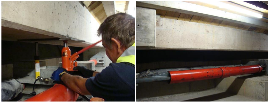
Figure 13: Left, equipment improvised to extract pin at right hand end from No. 21 damper. Right, No. 10 "spare" damper in place previously occupied by No. 21.
