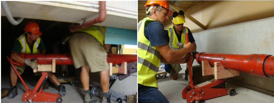
Figure 11: Left, damper No. 10 being rolled in through hatch. Right, damper turned parallel to installation position. In both pictures the damper is supported on wooden blocks fastened to floor jacks.
