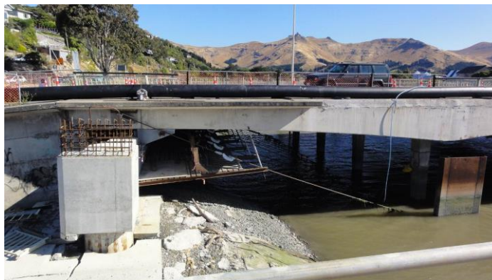
Figure 7: Tie rods installed to restrain the pier pile caps against further inward displacement.
