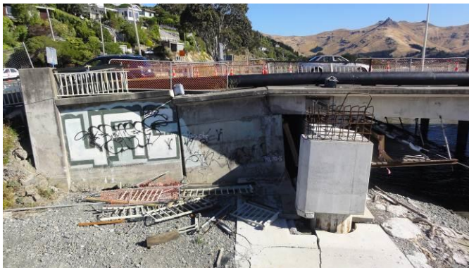
Figure 5: The Mt Pleasant abutment, displaced forward and rotated backwards about its raked piles founded on the bedrock; new bridge widening piles displaced outwards by lateral spreading.
