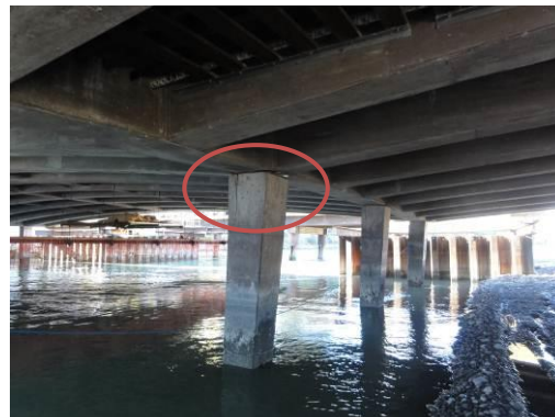
Figure 6: Pier columns rotated due to inward displacement of their supporting pile caps.
