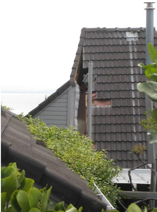
Figure 7: Superstructure distress caused by foundation failure on sloping ground (Beattie).
