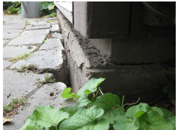
Figure 25: Example of a floor slab that has slipped sideways on the supporting foundation (Beattie).
