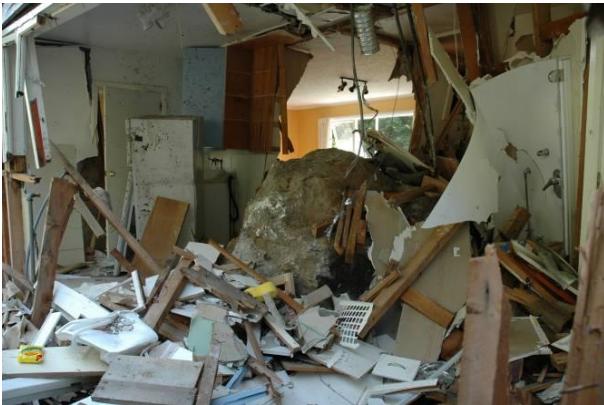
Figure 2: House damage in Heathcote due to rockfall (Carradine).
