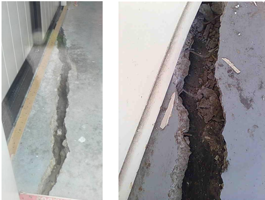
Figure 23: (Left) An unreinforced slab that has been pulled apart because of land spreading beneath (Beattie); (Right) A reinforced slab that has been pulled apart by land spreading beneath (Beattie)
