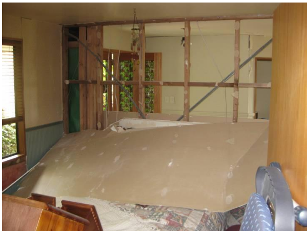
Figure 15: Failure of a generic plasterboard/metal brace combination (Beattie).
