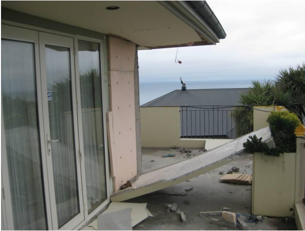
Figure 42: Failure of a concrete sandwich panel wall system (Beattie).
