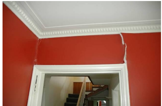
Figure 13: Buckled plasterboard in house in Heathcote Valley (Carradine).
