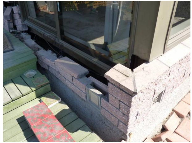
Figure 26: Example of a foundation wall that has pulled clear of the floor framing. Note how the veneer and foundation have pulled away from the framing at the corner (Beattie).
