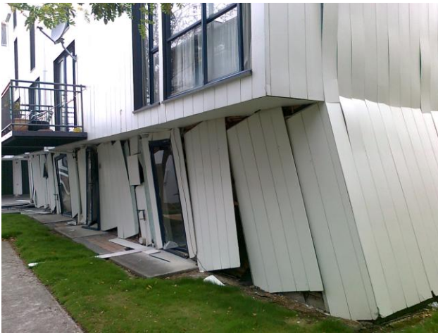
500 mm displacement, immediately after the earthquake (Structex).
