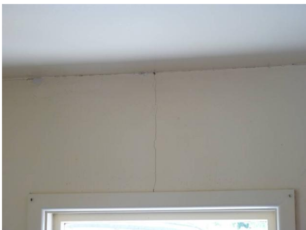
Figure 16. Cracking of a joint between fibrous plaster wall lining sheets (Beattie).
