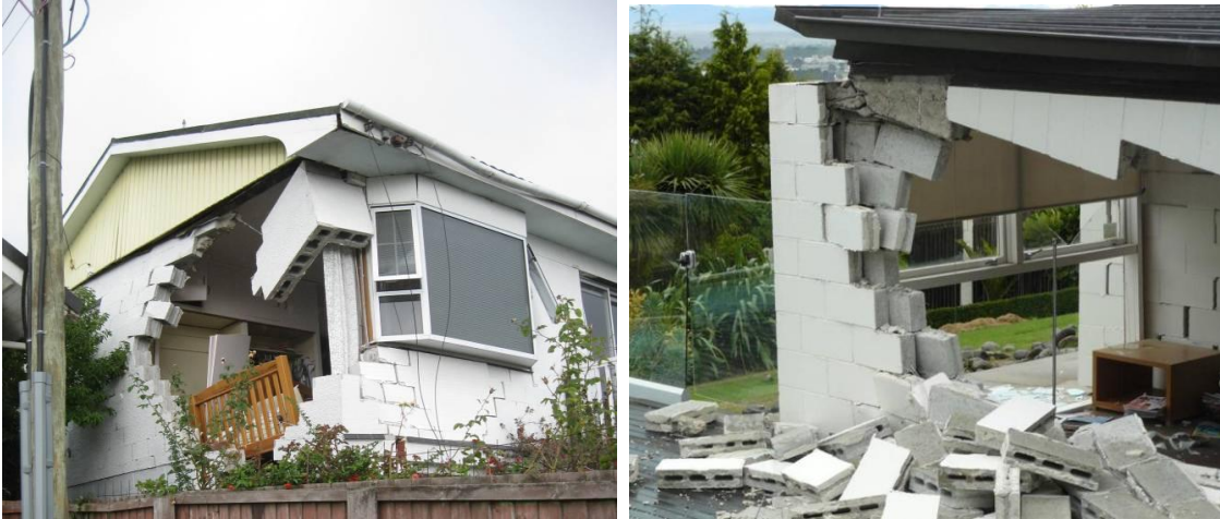
Figure 39: (Left) Collapse of unreinforced masonry exterior wall (Carradine), and (Right) Collapse of unreinforced masonry exterior wall (Morris).
