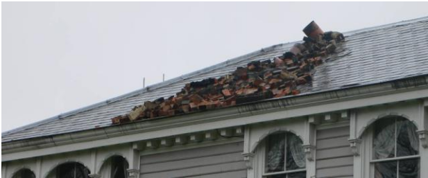
Figure 19: Fallen chimney bricks retained on a shingle roof with a solid timber substrate (Beattie).
