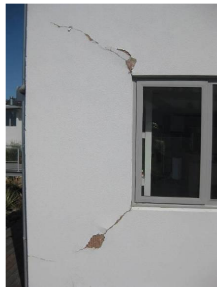
Figure 10: Typical cracking of an EIFS system (Beattie).
