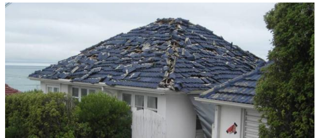
Figure 21: Dislodged heavy roof tiles on a hillside property (Beattie).
