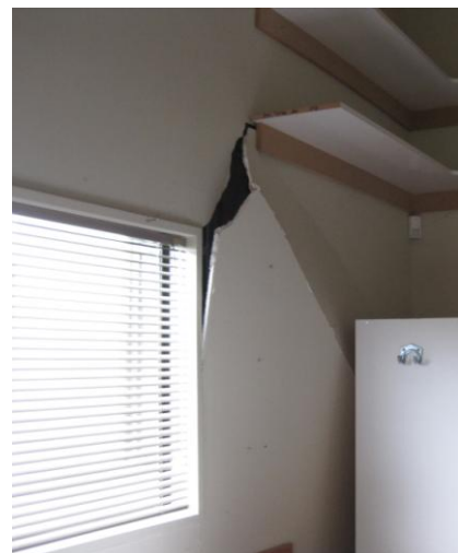
Figure 35: Damage to plasterboard bracing sheet glued to steel studs with no screws.
