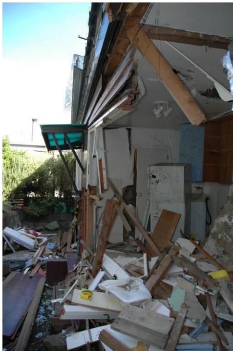
Figure 3: House damage in Heathcote due to rockfall (Carradine).
