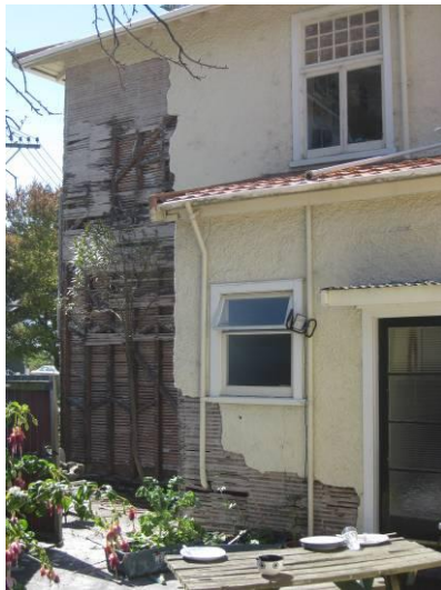
Figure 12: Detached lath and plaster from an exterior lath and plaster system (Beattie).
