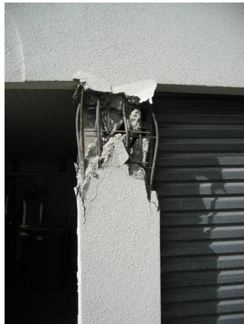
Figure 41: Compression failure of tilt-panel concrete house (Carradine).
