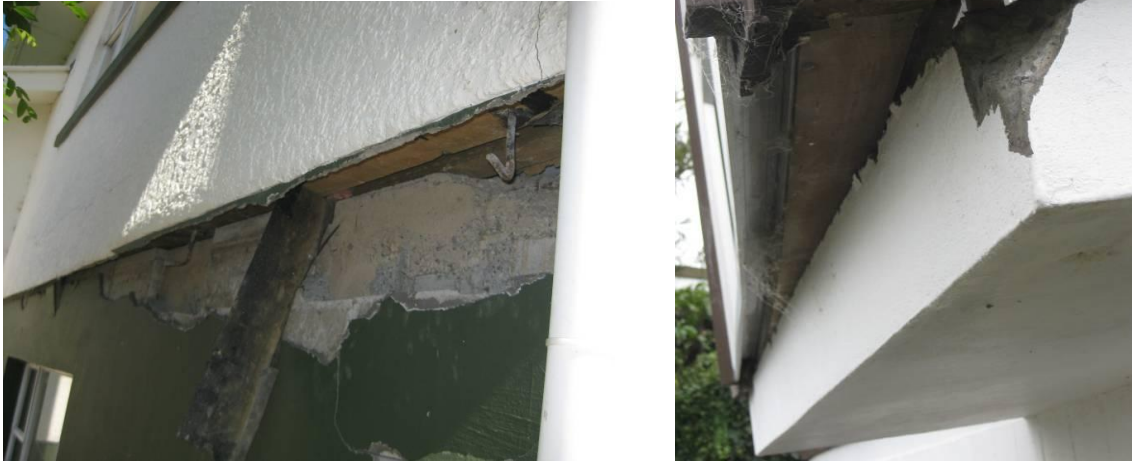
Figure 28: (Left) Bottom plate anchors that have torn out of the unreinforced concrete foundation wall; (Right) No apparent connection between the plate and the concrete slab (Beattie).
