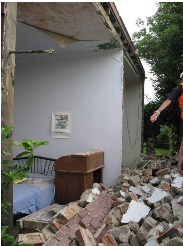
Figure 37: Failure of brick fire wall near city centre (Carradine).
