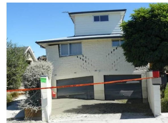
Figure 9. Veneer damage due to lateral spreading and differential settlement (Buchanan) and due to differential settlement (Morris).
