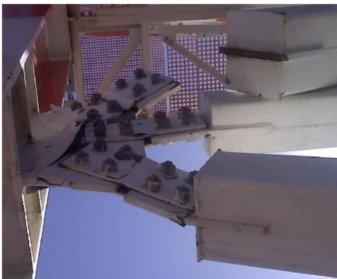
Figure 5.12a: Fractured steel bracing cleat. (Photo: Carlos Aguirre).
