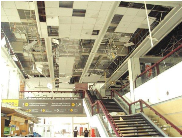
(a) Post earthquake (Photo: G. Segovia).
