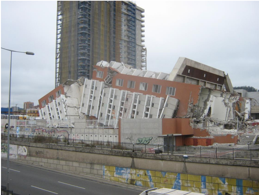
Figure 5.3e: Catastrophic failure of the multi-storey “Alto Rio” apartment block in Concepción. (Photo: Hugh Cowan).
