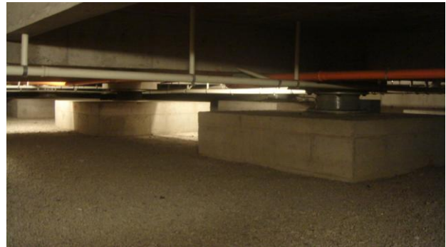
Permanent offset of lead rubber bearing Catholic University of Chile building.
