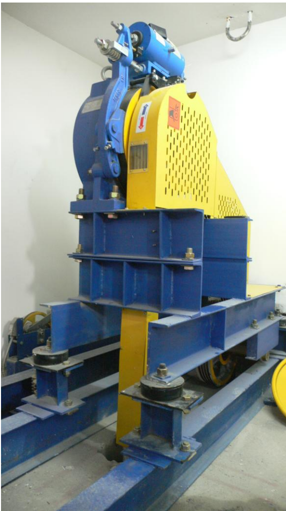
(e) Motor still well restrained.
