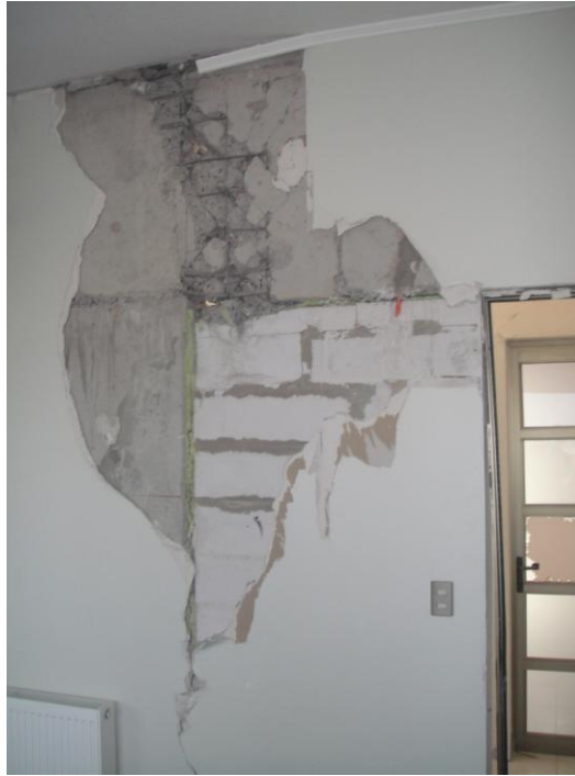
Figure 5.8a: Seismic separation. (Photo: Peter Smith).
