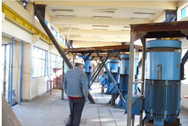
Figure 8.9: Propping and steel frames built to protect pumps in ESSBIO water plant. (Photo: C. Oyarzo-Vera).
