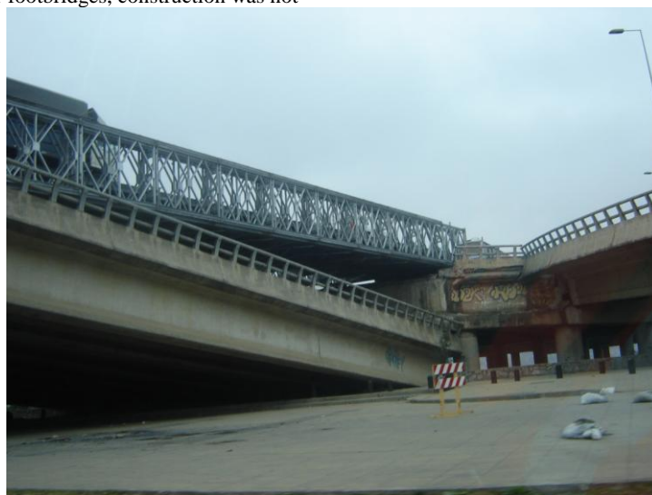
Figure 8.2: Bridge deck collapse and a bailey span repair in Concepción. (Photo: Graeme Lawrence).
