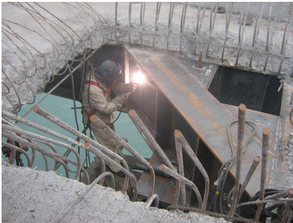
Figure 8.8: Repairs to the north pier at Coronel Port consisted of driving new steel piles and welding them to the existing deck structure. (Photo: Hugh Cowan).
