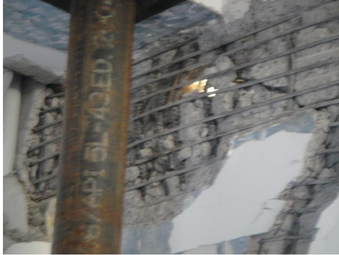
Failed shear wall in apartment building shown to the left, Santiago.
