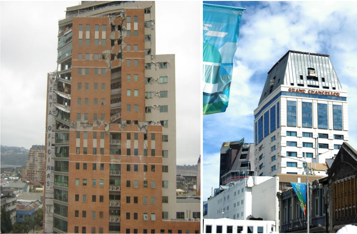
Figure 5.3b: The partial collapse of large commercial buildings, such as the O'Higgins Tower of Concepción, Chile (left) and the Grand Chancellor Hotel of Christchurch, New Zealand (right) highlights the vulnerability of surrounding areas to prolonged denial of access and business interruption. (Photos: Hugh Cowan).
