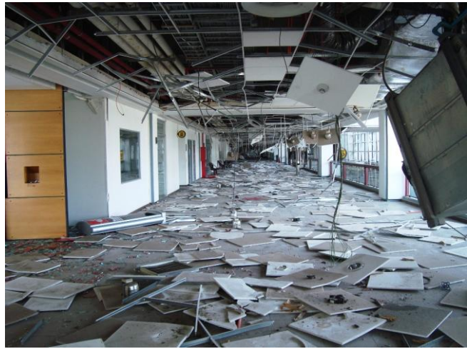
(b) Post earthquake (Photo: G. Segovia).
