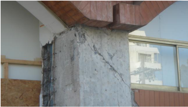
Low-rise commercial building with shear failure of columns due to non-isolation of infill walls, Valparaíso.
