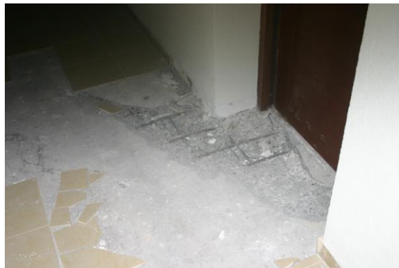
Figure 5.3k: Floor slab shear damage at end of shear walls in an apartment building in Concepción. (Photo: Clark Hyland).
