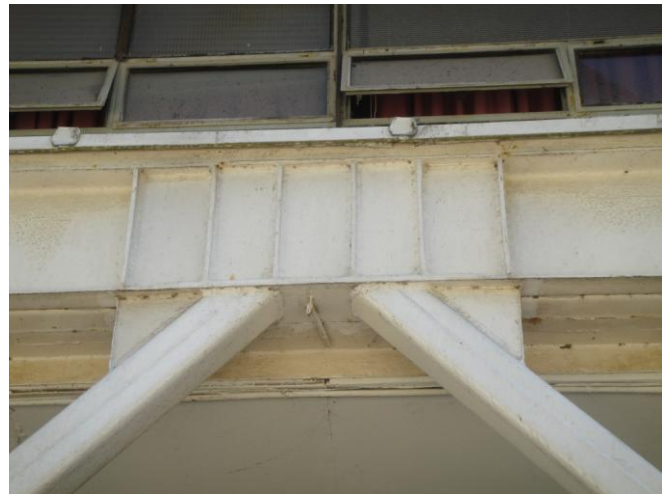
Unyielded steel active link in three-storey building at University of Concepción.
