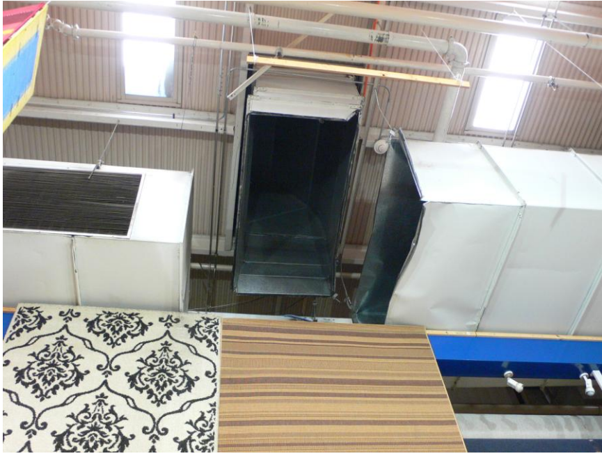
Figure 5.7d: Santiago International Airport - air handling fan missing and damaged ducting. (Photo: Graeme Beattie).
