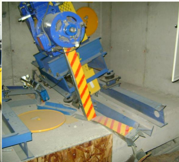
(f) Motor mounting has failed.
