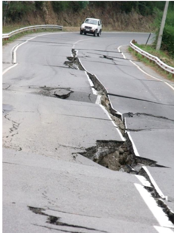
Figure 8.1: Damaged road near Concepción. (Courtesy of A. García).
