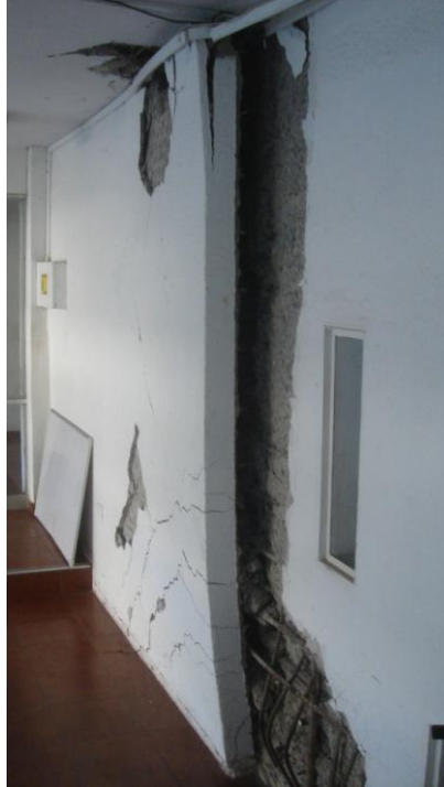
Figure 5.4a: Shear wall delamination – Festival Apartment Building. (Photo: Peter Smith).
