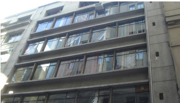
Pounding between tower and podium of Direccion Regional Santiago Centro.
