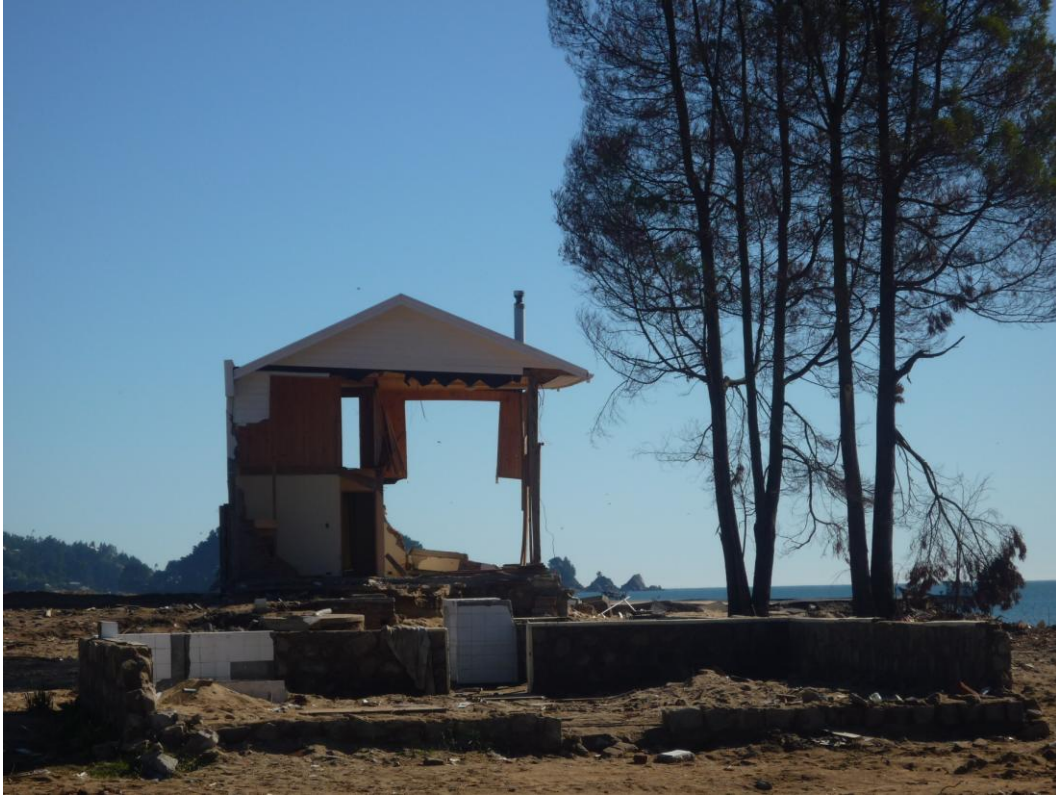
Figure 2.2c: Complete destruction of coastal dwellings where the tsunami came ashore at Dichato, north of Concepción. (Photo: Katherine Hill).
