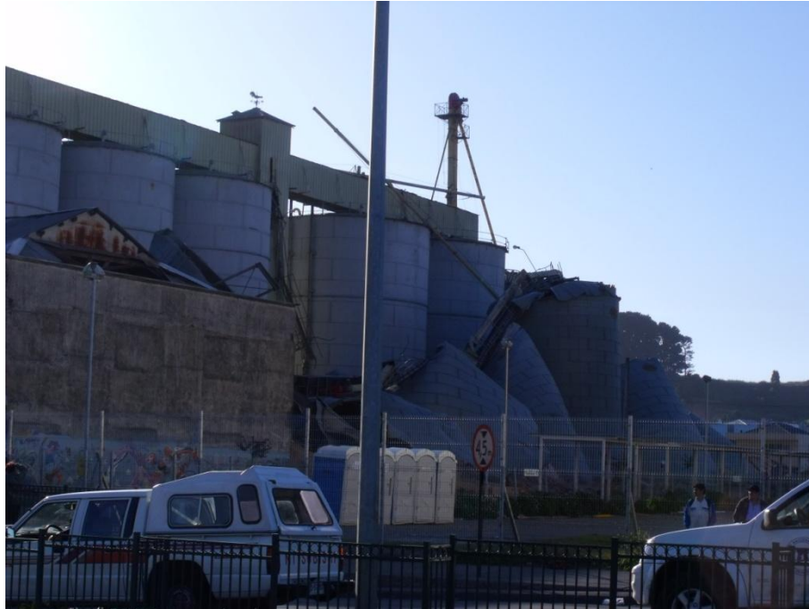
Figure 5.12c: Collapsed grain Silos in Concepción. (Courtesy of A. García).
