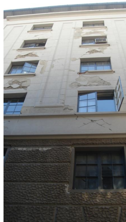
Damaged spandrels to early reinforced concrete building in central Santiago.
