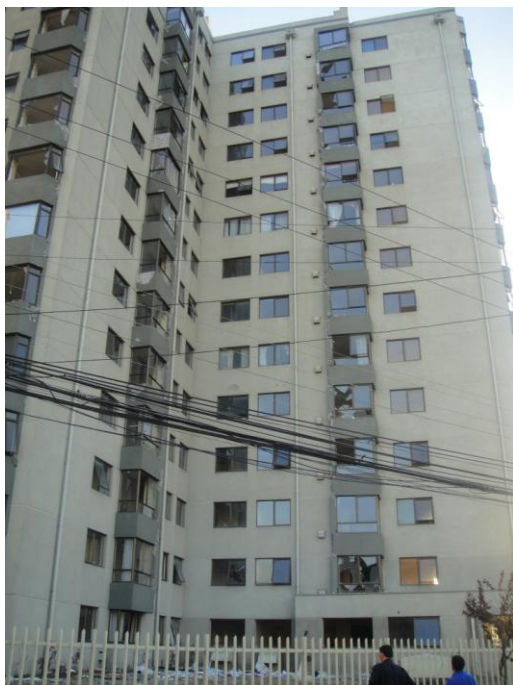
Damaged tower to Plaza Mayor building.
