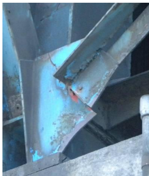
Figure 5.12b: Fractured steel gusset plate connected to a chevron-braced frame. (Photo: Carlos Aguirre, UTFSM).
