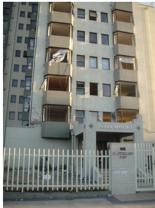
Damaged tower to Plaza Mayor building.
