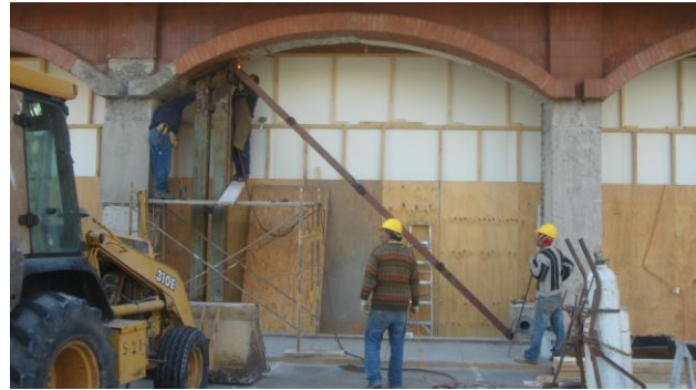
Low-rise commercial building with shear failure of columns due to non-isolation of infill walls, Valparaíso.
