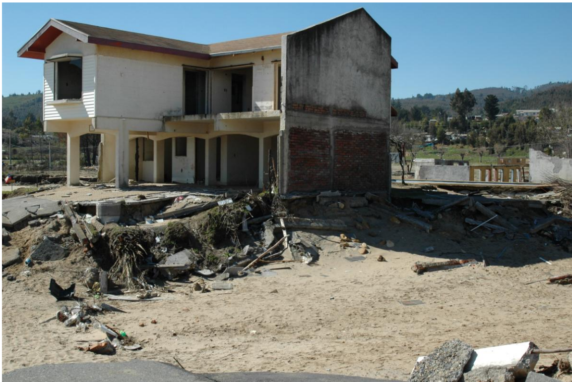
Figure 2.2d: Receding water caused severe scouring of foundations beneath coastal structures at Dichato. (Photo: Hugh Cowan).
