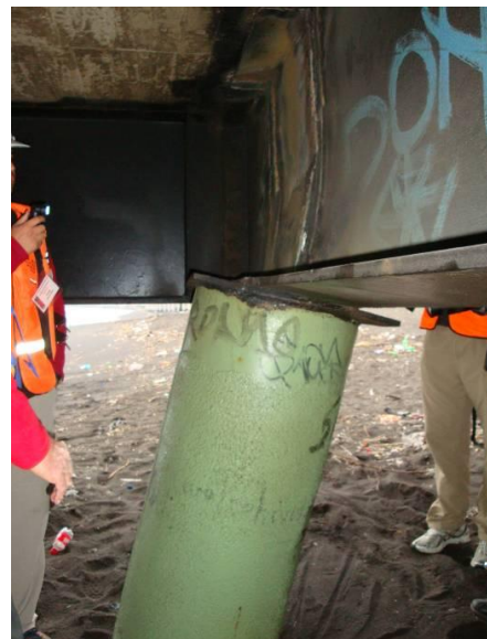
Figure 8.7b: Pile head deformed due to abutment shunting caused by liquefaction. (Photo: Clark Hyland).
