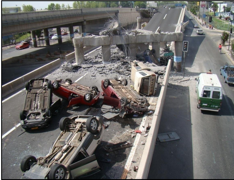
Figure 8.3: Collapse of a bridge deck on the Santiago ring-road “Vespucio Norte”, due to lateral rotation of the obliquely-seated deck and absence of diaphragms. (Photo: Ministerio de Obras Públicas).
