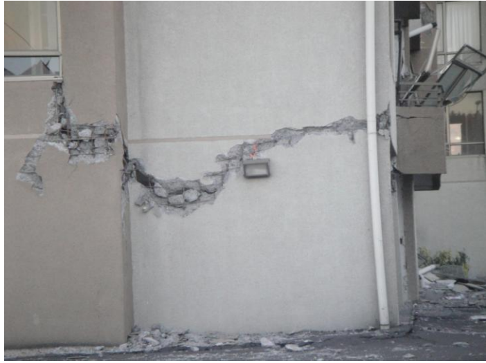
Shear wall failure, Plaza del Rio Apartments, Concepción.
