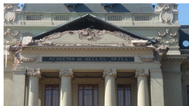
Failed parapet Academia de Bellas Artes, Santiago.
