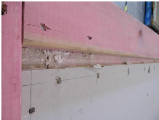
(c) Screw head rotating due to slip between sheets and framing
