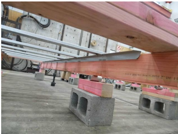
Figure 5: Underside of ceiling diaphragm specimen during construction showing joists, battens, Rondo N18 angles and supporting rollers.
