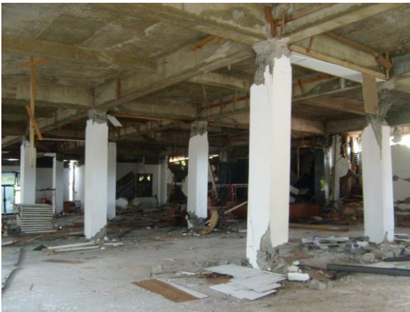
b) Plastic hinging of columns of an open bottom storey.
