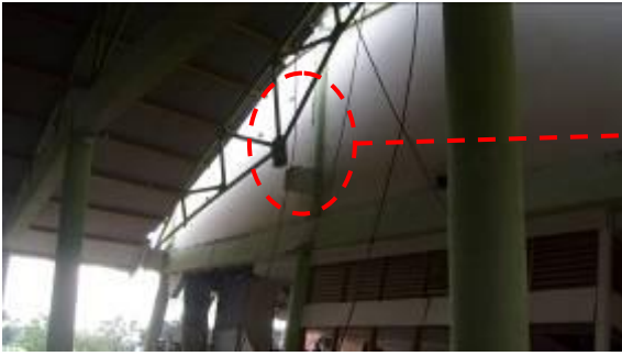
a) Anchor and roof bracing ties failure.
