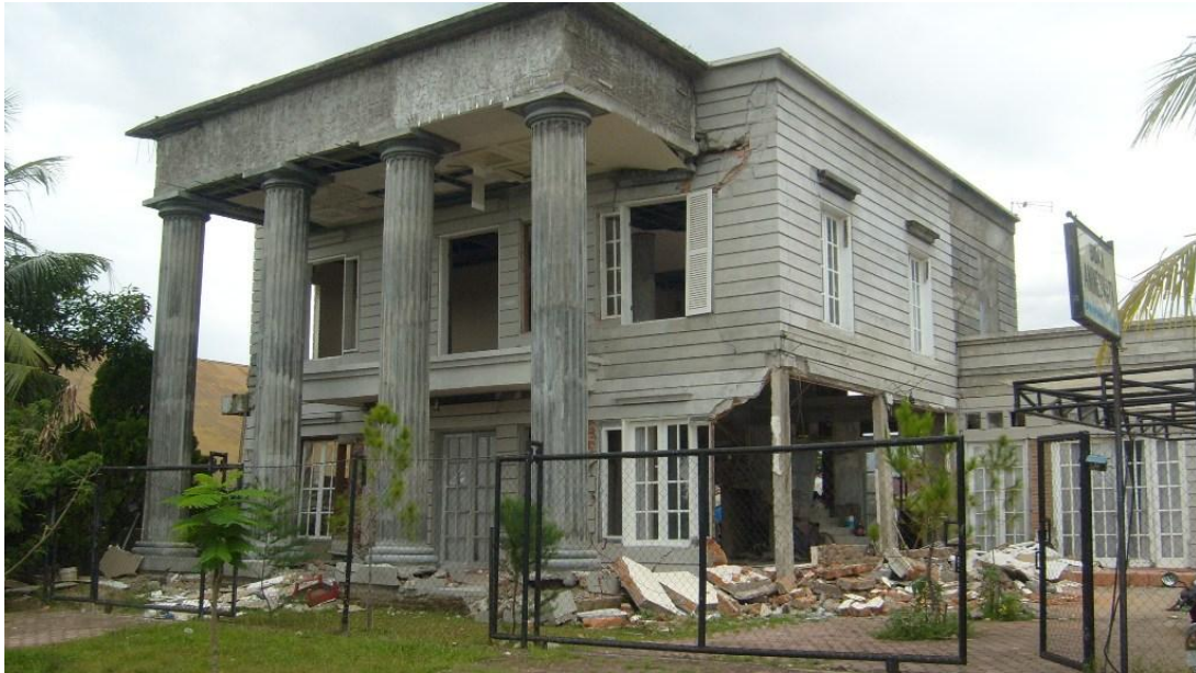
b) Out-of-plane failure of a brick wall in a building with practical columns and beams.
