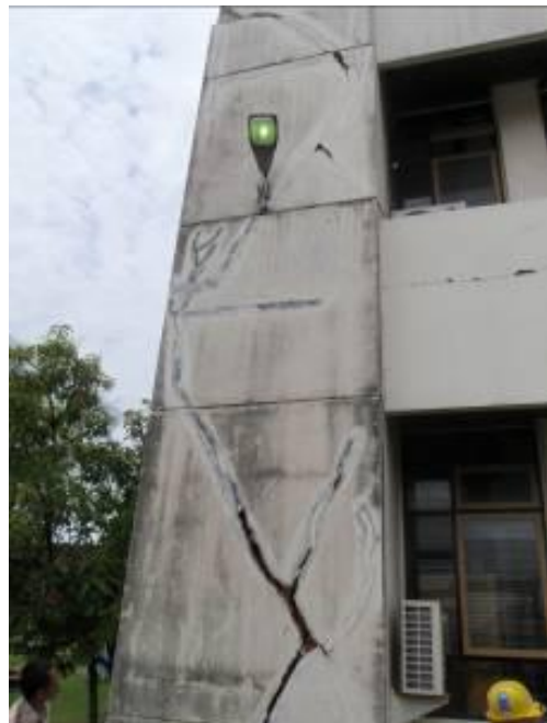
Figure 5.7: Diagonal cracks in a pier. This building was damaged in the 6 March 2007 M6.4 earthquake, but the building was not strengthened and the cracks were just covered.
