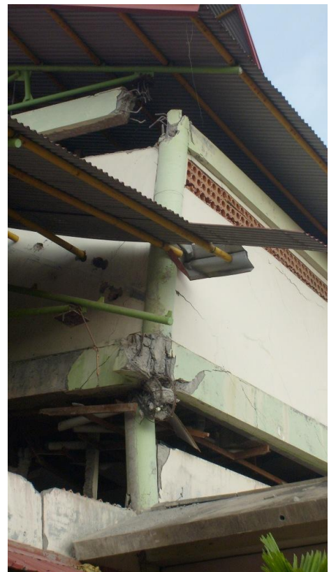
d) Beam bar anchorage failure (at roof level) and crushing of column in the bus terminal building.
