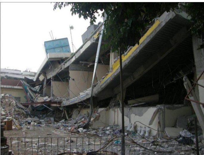
f) Failure of columns leading to failure of high-bond floor.
