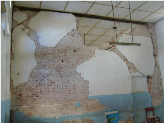
a) Diagonal shear crack combined with out-of-plane failure of an unreinforced brick wall in a school (note separation of in-plane and face loaded walls).
