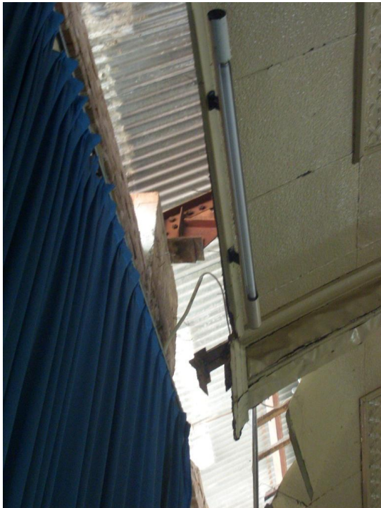
Figure 6.30: Failure of anchors between a steel roof truss and concrete column in an old church.
