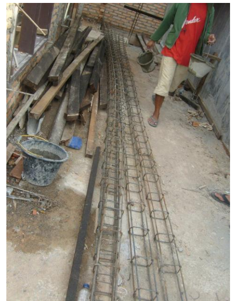
c) Reinforcement ready for a practical beam. More stirrups would make a big improvement.
