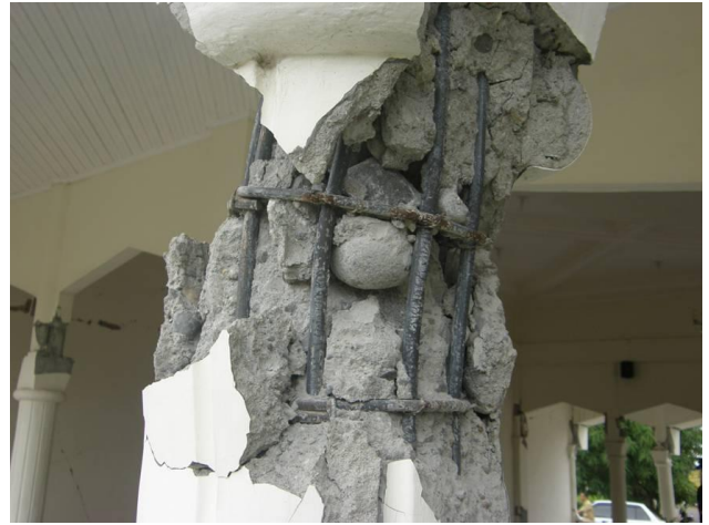
Figure 5.5: Segregation of concrete and large pebbles/cobbles in the concrete. Note 90° hooks and wide spacing of stirrups.
