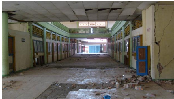
Figure 3.5: Differential settlement of foundation and floors of the Padang Bus Terminal has strained and deformed the entire building.
