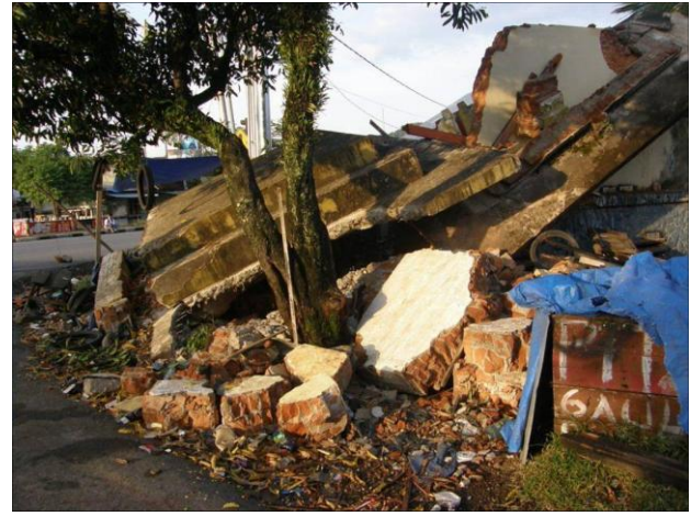
b) Total collapse of a similar unreinforced masonry building.
