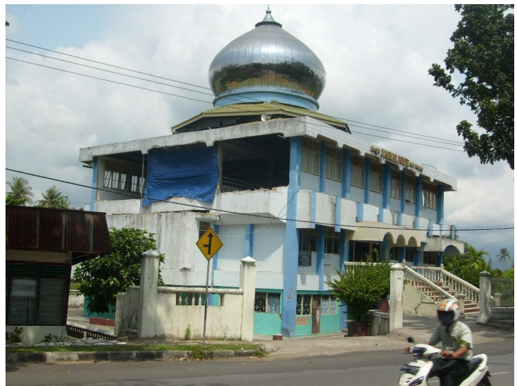
c) Out-of-plane failure of infill walls.
