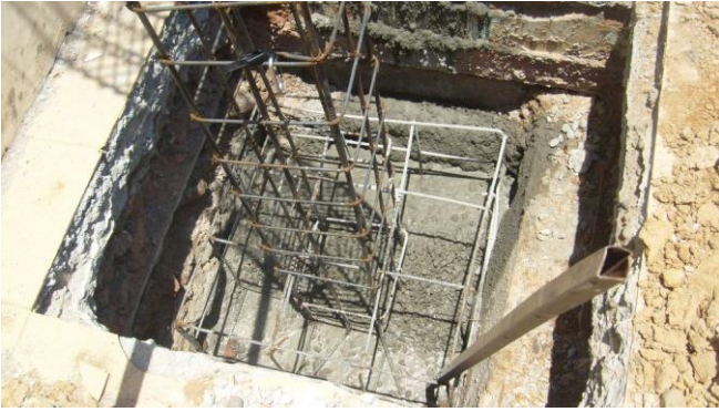
Figure 5.4: A typical isolated foundation pad for a RC frame building. Note inferior quality of concrete and the wide spacing of stirrups with 90° hooks.
