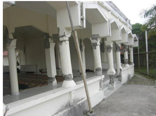
c) Column hinging at top and bottom. The building survived due to the alternate gravity load-carrying system provided by the walls. Note the large rotation of columns imposed by shortening of columns due to the sill wall.
