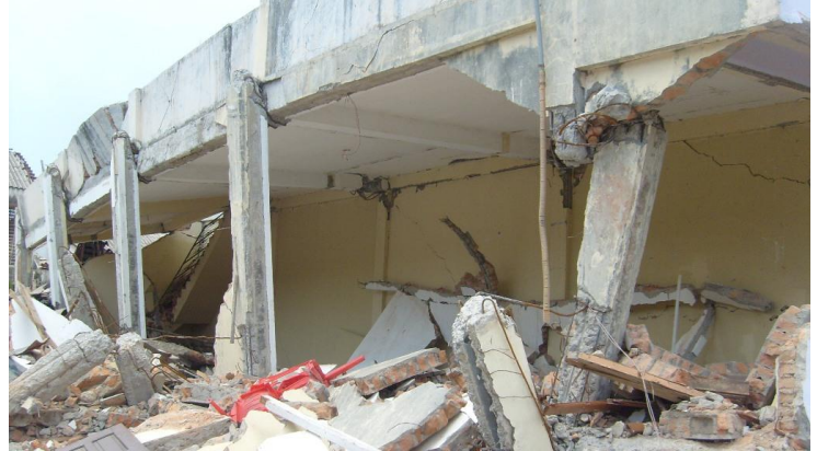
b) Cold-joint problem.
