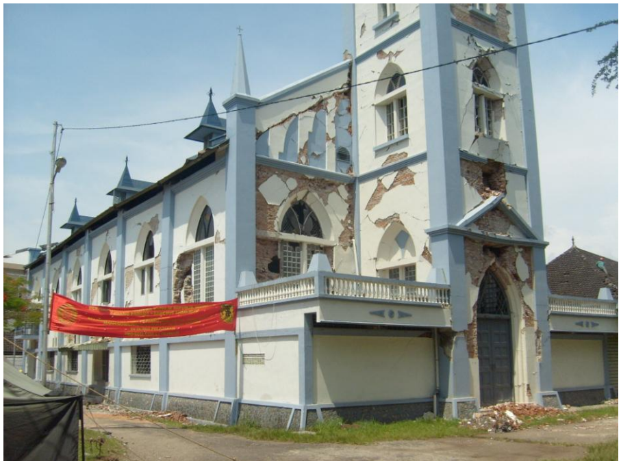
Figure 6.22: A badly damaged Dutch-era masonry brick church building with a recently added internal RC frame and slab mezzanine floor—which probably prevented complete collapse.
