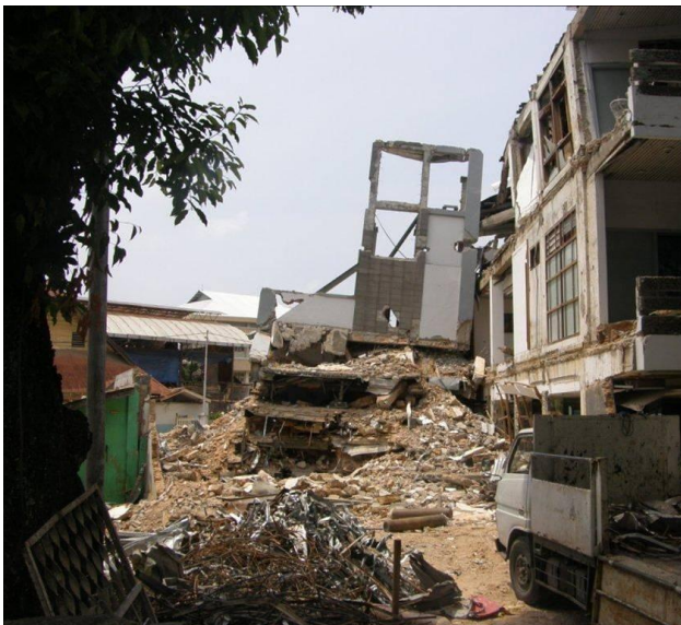
a) Pancaking after weak axis column bending failure.
