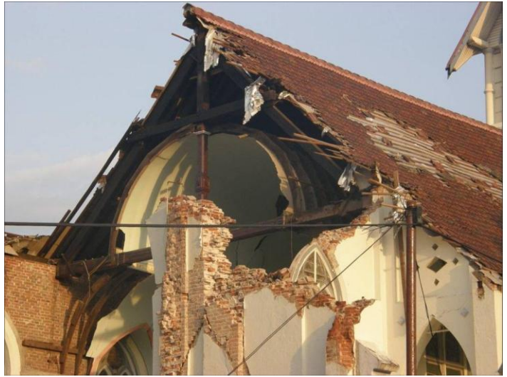
b) An old masonry brick church barely survived the earthquake. The roof survived because of alternative load paths.
