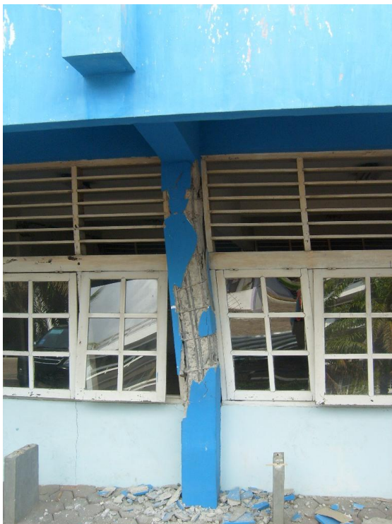
Figure 6.7: Short column failure. Note how the timber window frame has influenced the failure.
