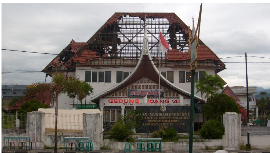
Figure 7.1: Shedding of untied tiles.
