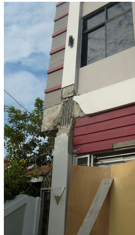
e) No stirrups in beam-column joint.
