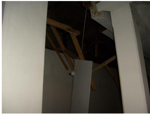
Figure 7.3: Damage to false ceilings was common.
