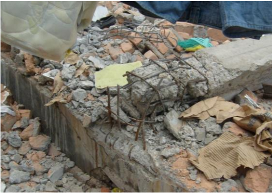
a) Failure of column bar splicing.
