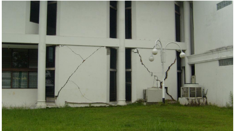
b) Diagonal failure of infill walls separated from columns.
