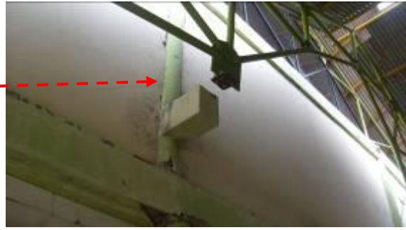
b) Anchor plate failure (note the plate was anchored to an adjoining building).
