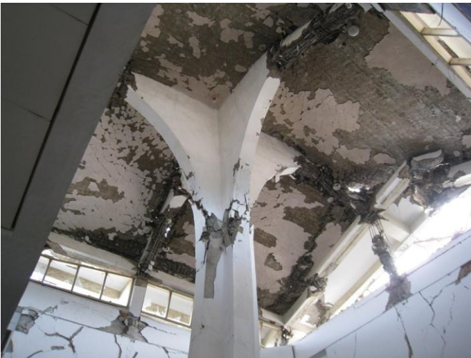
c) Failure of column due to sudden change of stiffness.
