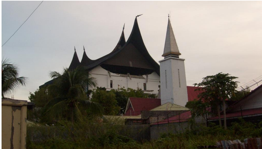
Figure 7.2: Tilting “pinnacle” and toppled gable wall.
