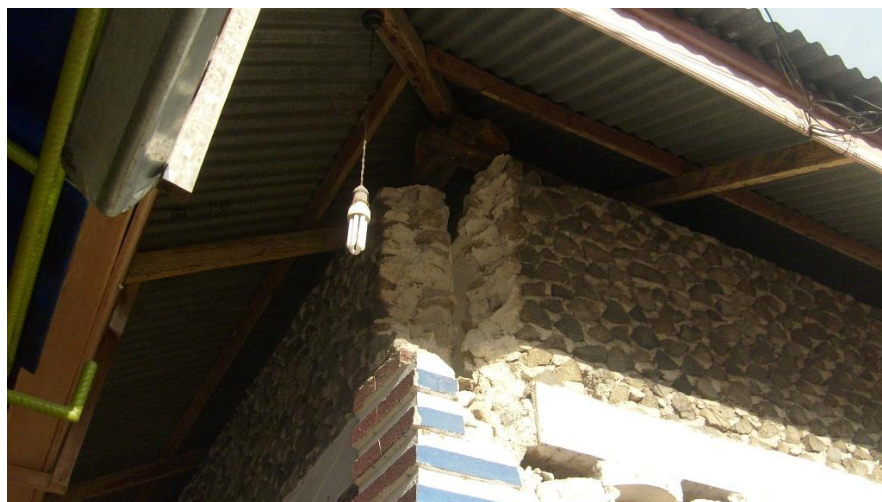
Figure 6.17: Corner failure (note lack of connection between walls).
