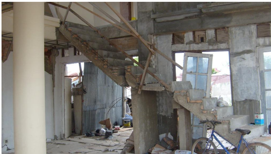
Figure 6.33: Compression failure of a waist slab.
