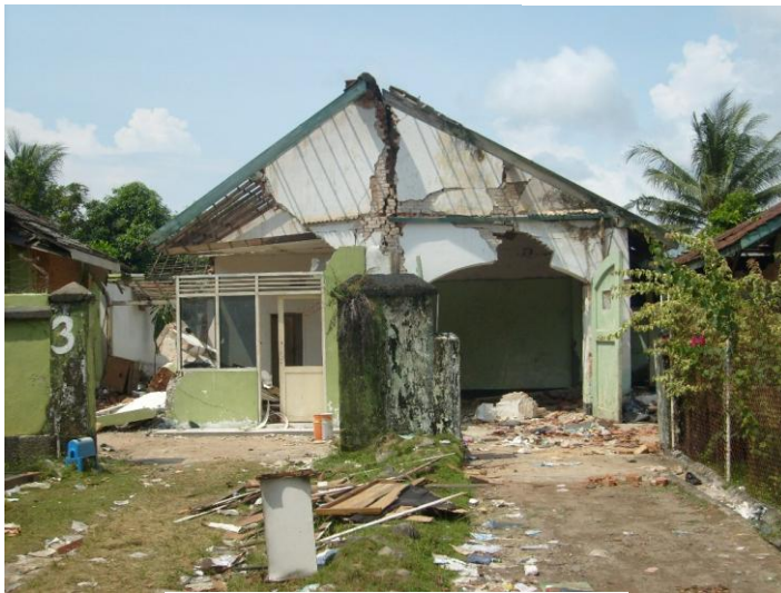
c) Vertical cracking of a house wall.
