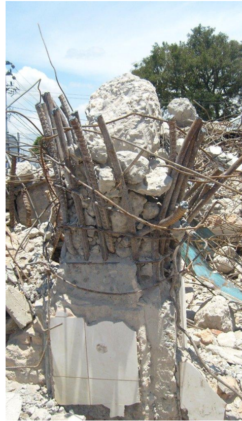
c) Mixing of plain and deformed reinforcing bars.
