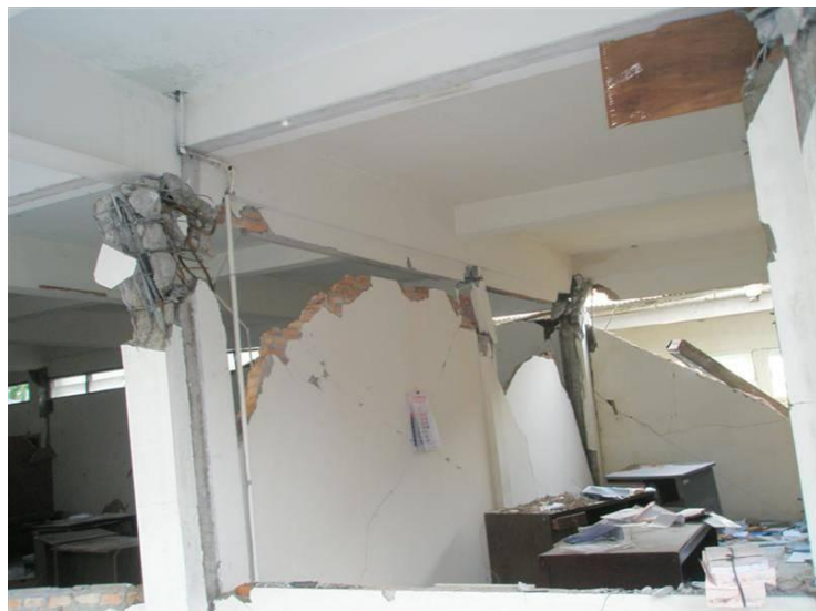
c) Column failure due to shear imposed by infill wall structure.
