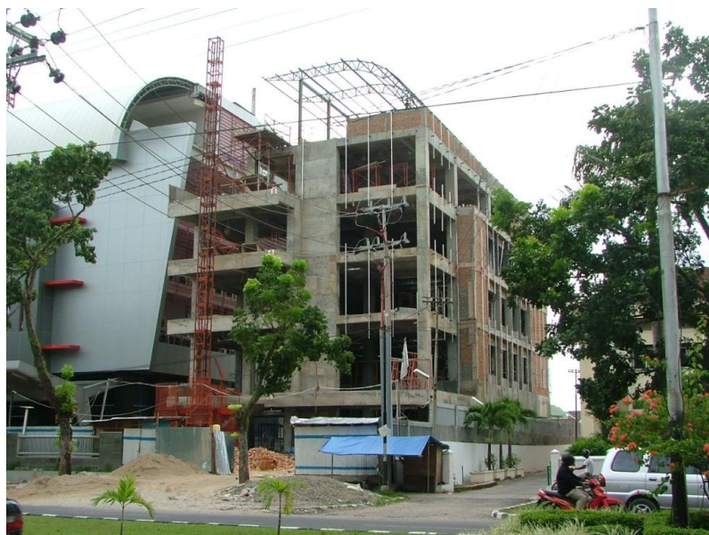
Figure 6.18: A rare example of a new RC frame building with concrete shear walls under construction.
