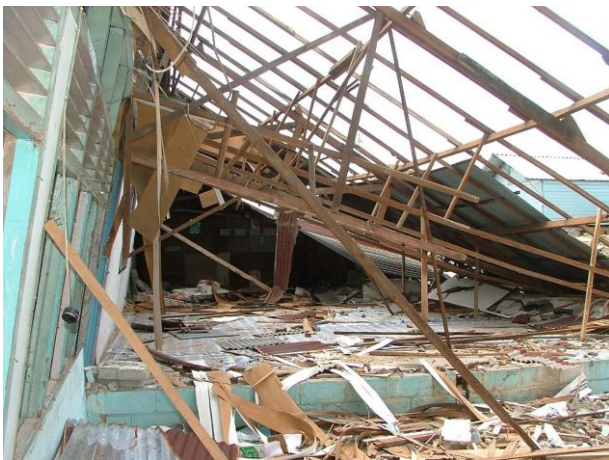
c) Failure of a poorly connected roof due to loss of support.
