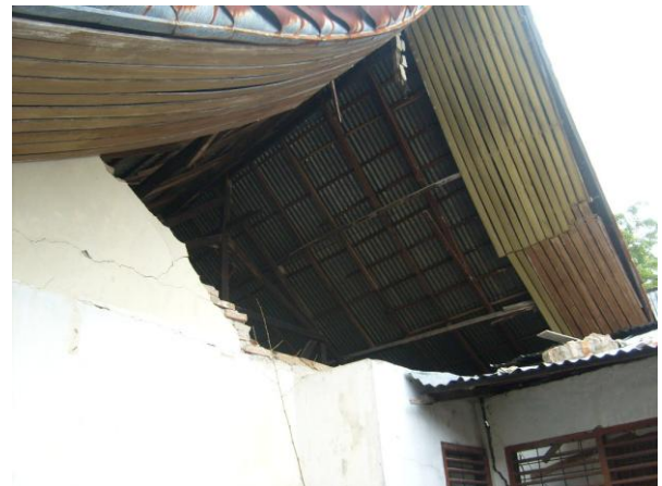
d) Toppling of a gable wall.
