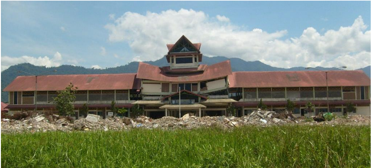
Figure 6.20: Padang's bus terminal building suffered extensive damage due to differential ground settlements and soft storey collapse of the central block. Note destruction of the second storey; roof ridge should be horizontal.
