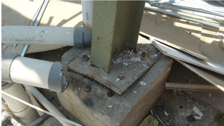
Figure 5.6: Missing nuts, bending of base plate resulting in large rotation of the column base.
