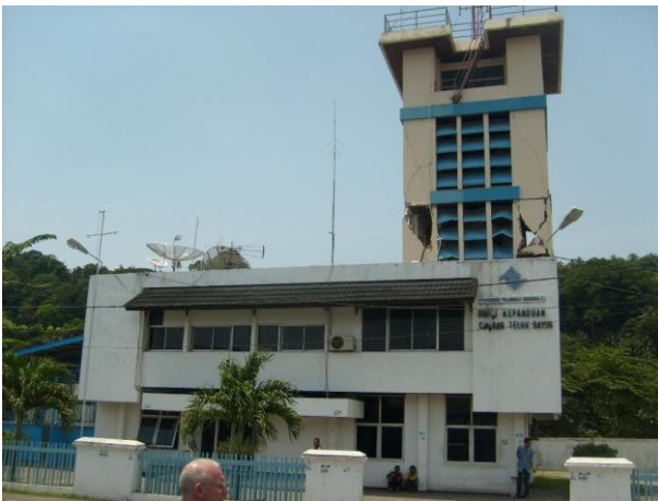
Figure 6.2: Damage due to shaking amplification.
