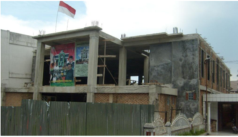
a) A typical RC frame building under construction with brick masonry infill panels. Note the deficient length of column reinforcement for future extension.
