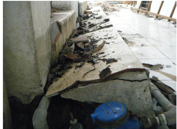
Figure 3.2: Settlement damage to a large building due to liquefaction and expulsion of water and fine sand. Buildings on sand strata near drains, creeks and rivers suffered from failure due to lateral spreading of soil. In one case half the length of a classroom building had dropped 800 mm compared to the other half.
