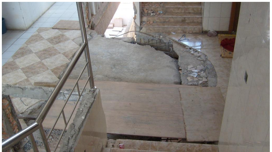
Figure 6.5: Rupture of a slab bridging two buildings (see Figure 6.3 for layout of the buildings).
