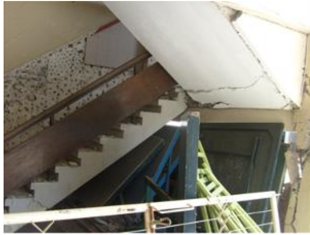
Figure 6.32: Compression-flexural crack between waist slab and supporting beam.
