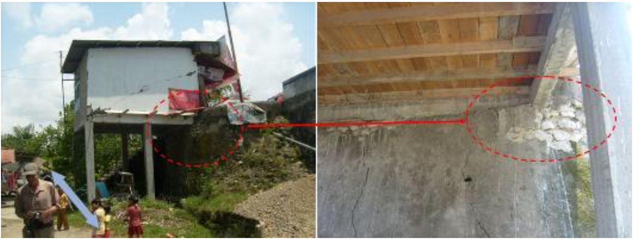
Figure 6.6: Building on stilts (arrow shows direction of shaking).
