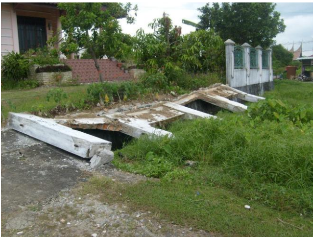
a) Toppled boundary walls were common.
