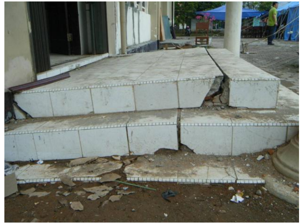
Figure 3.1: Settlement damage to building steps.
