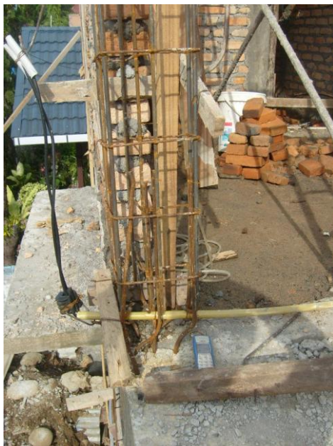
d) Bent bars at the column base.
