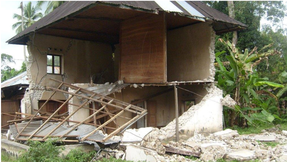
Figure 6.16: Partial collapse of a stone masonry house building due to out-of-plane toppling of walls (note lack of connection between structural components and shear failure of piers).
