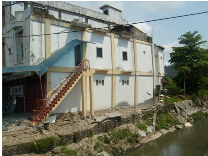
Figure 3.4: Settlement of ground surrounding a building due to lateral movement and rotation of a retaining wall.
