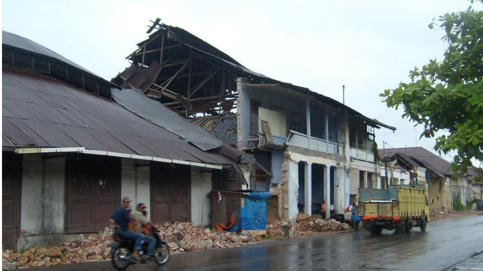
a) A building with out-of-plane collapse of walls.
