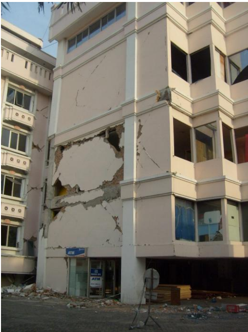
a) Wall panel is stable, even after severe damage.
