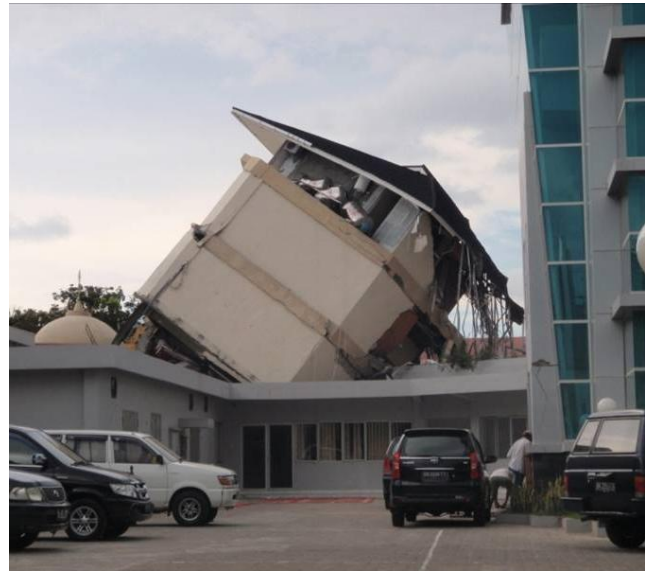
b) Building collapse due to column failure.
