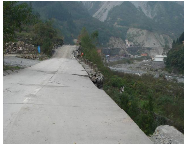
Figure 133: Ramping up road across fault rupture, near Qingping.
