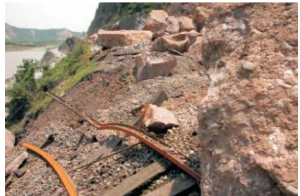
Figure 123: Railway line destroyed by landslide.
