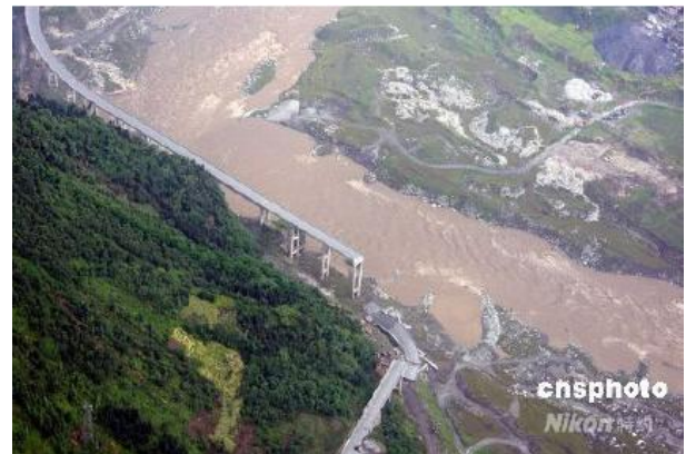
Figure 79: Baihua Bridge after the earthquake.
