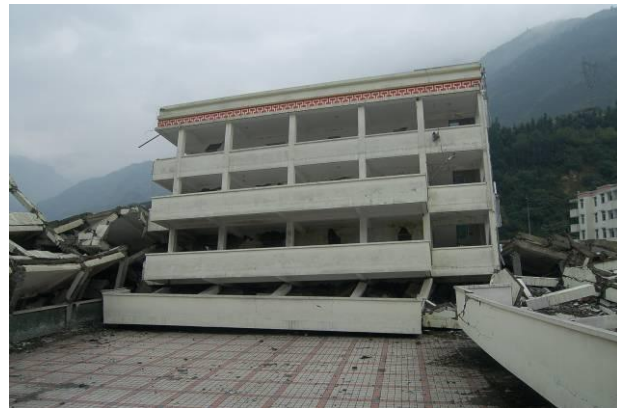
Figure 61: Soft story - Classroom Block 2.
