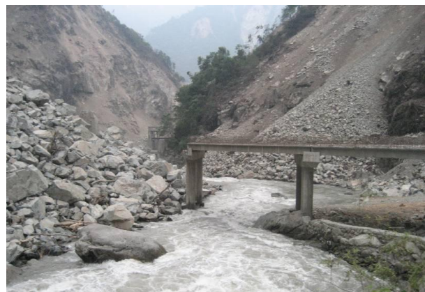
Figure 129: Landslide destroying bridge access across river.
