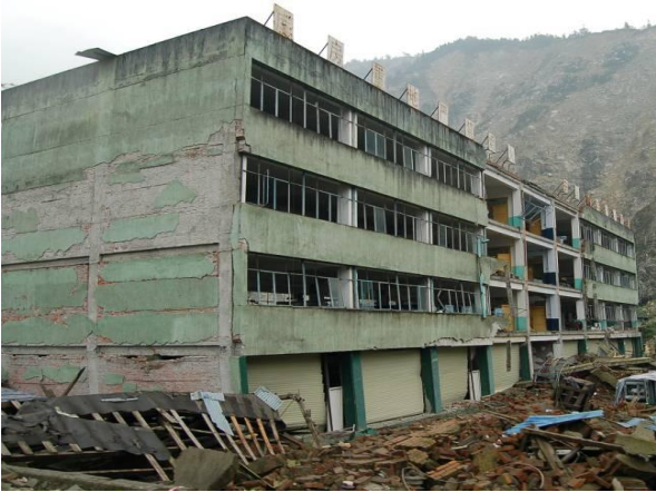
Figure 53: Reinforced concrete framed structure with masonry in fill with soft story failure at the bottom level.
