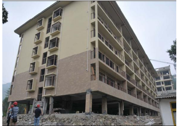
Figure 76: Soft story at the bottom, large change in structural stiffness vertically.
