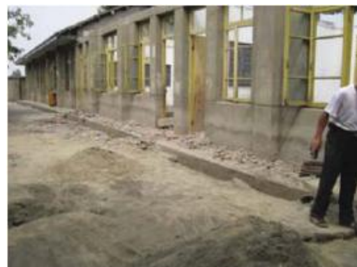
Figure 108: Liquefaction at Zhongxing Middle School in Dujiangyan City (after Longwei et al , 2009).
