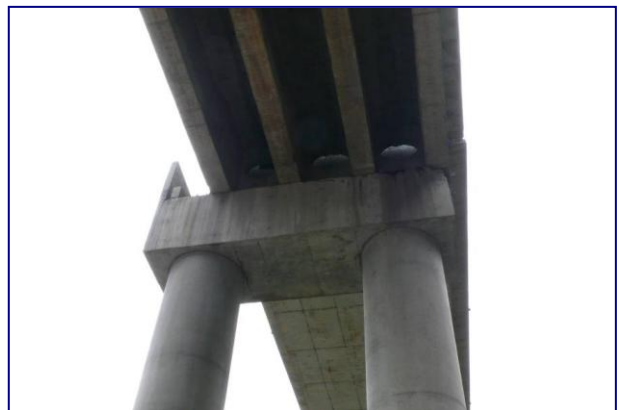
Figure 87: Lateral displacement of bridge deck at bridge Section 3.
