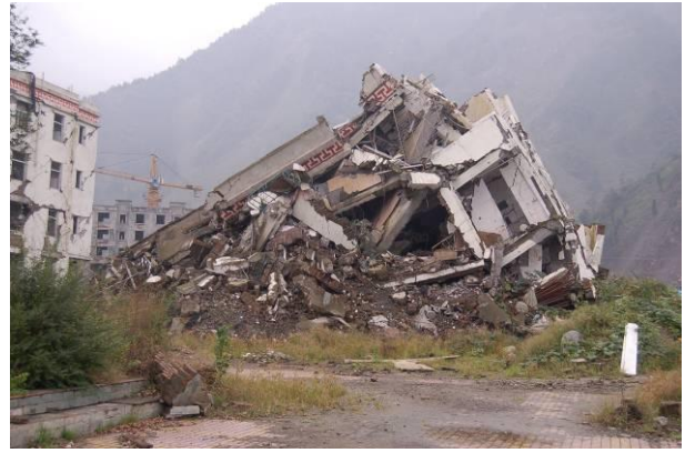
Figure 59: Dormitory Block – complete collapse.
