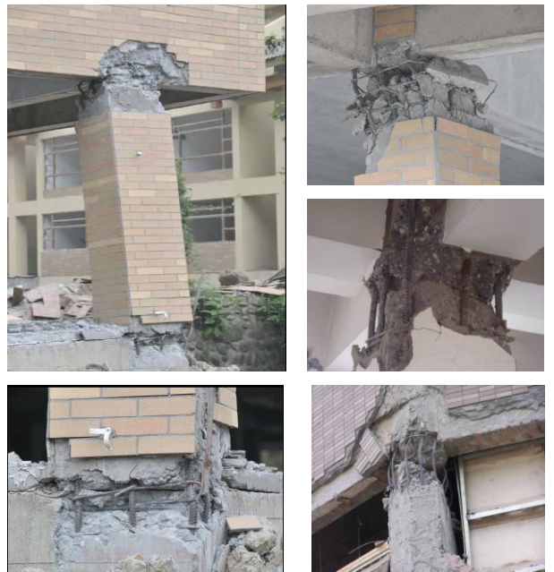
Figure 77: Inadequate transverse reinforcement in the columns.
