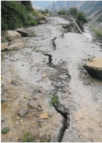
Figure 125: Loss of road platform due to underslips.
