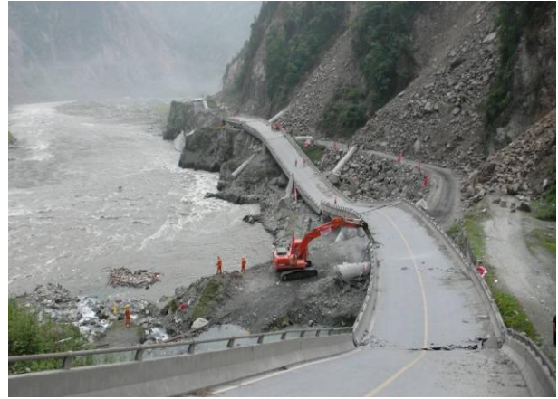
Figure 132: Partially collapsed Baihua bridge blasted down with explosives to make access along Highway 213.
