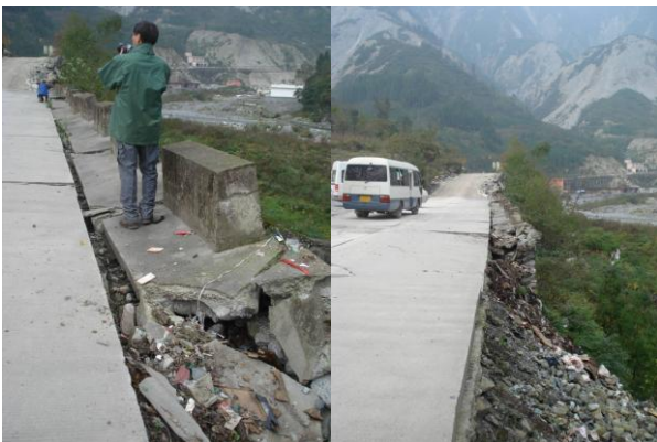
Figure 115: Section of retaining wall that has displaced up to ~200 mm, and section that collapsed adjacent to fault rupture near Qing Ping.
