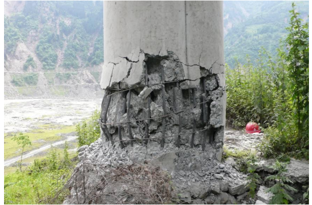
Figure 84: Shear failure, buckling of main reinforcing bars, spacing of stirrups in excess of 400 mm.
