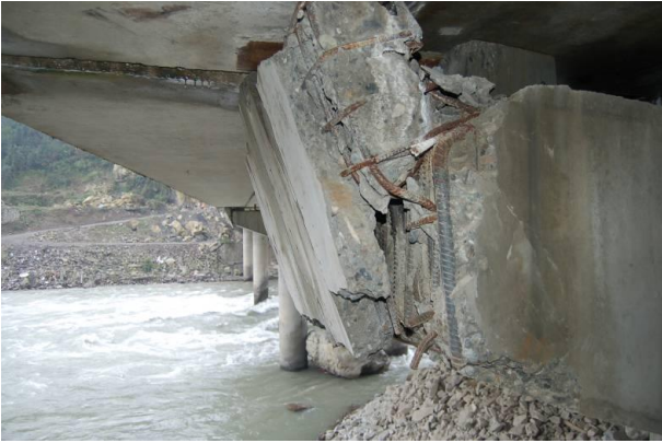
Figure 94: Damage to shear key due to the horizontal inertia force from the deck.
