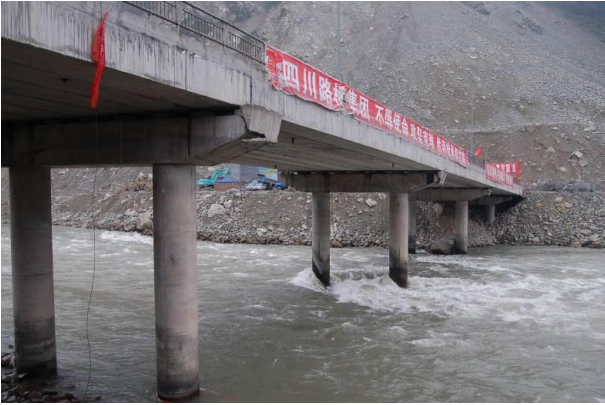
Figure 93: A bridge that runs parallel to the fault rupture near the Epicentre, suffered considerably less damage, large movement of the deck, up to 1 m horizontally .
