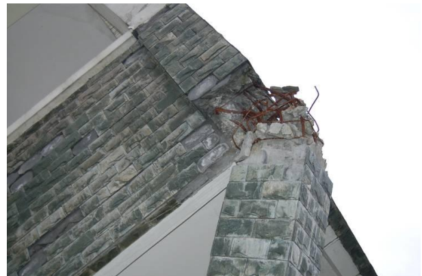
Figure 62: Lack of column transverse reinforcing.
