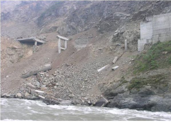
Figure 130: Viaduct bridge destroyed by landslide.
