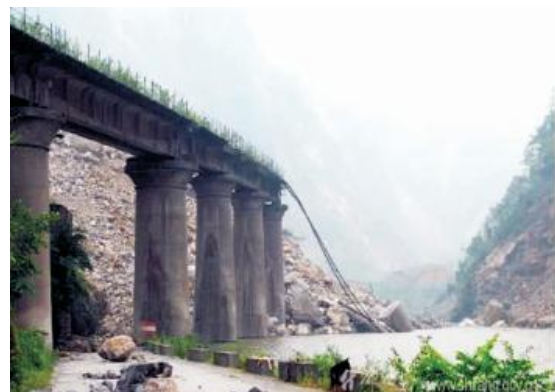
Figure 124: Railway bridge collapse due to landslide.
