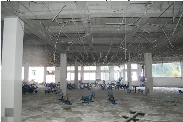
Figure 70: The school dining hall, minor structural damage but severe damage to the architectural fixtures.
