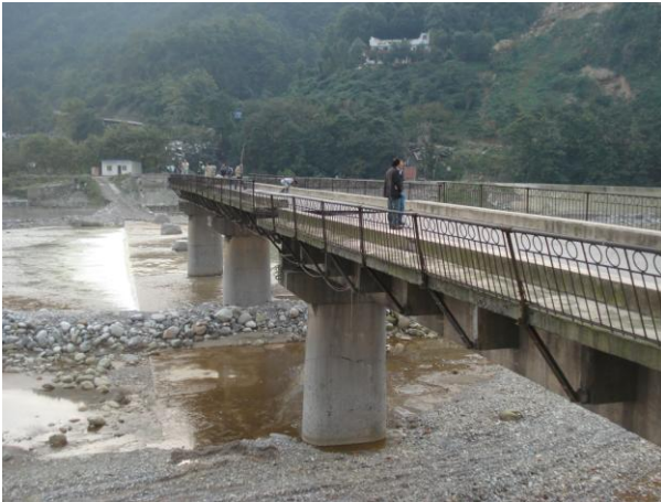
Figure 105: Bridge collapse due to fault rupture.
