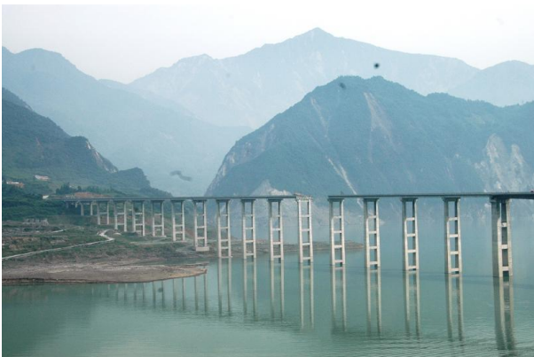
Figure 89: Loss of seating at span no. 10.
