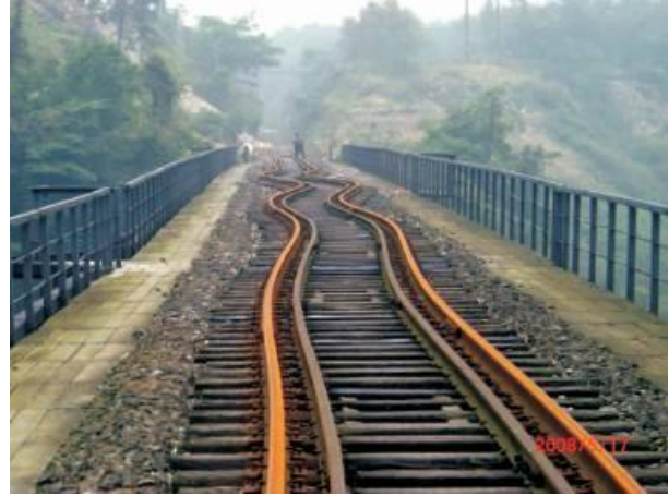
Figure 122: Damaged railway line.
