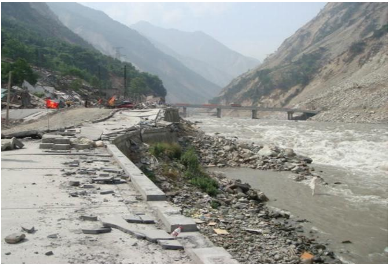
Figure 15: The Yingxiu-Beichuan fault cut through the river bank road north of the Yingxiu Township. The earthquake caused vertical and horizontal displacements of 2 m and 1.7 m, respectively, across the fault. (From Chen Yuntai, Chinese Academy of Sciences.)
