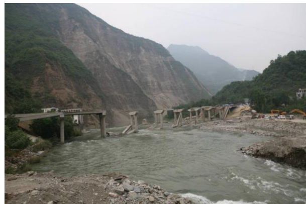
Figure 128: Loss of access from collapse of river bridge.
