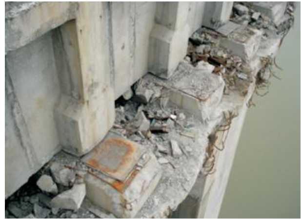
Figure 90: Close up view, no linkage bolts.
