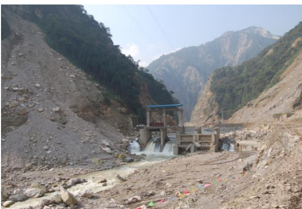
Figure 103: Irrigation control structure on Mianyu River upstream of Hanwang. Much of damage believed to be from partial breach of Yi Ba Dao landslide-dammed lake.
