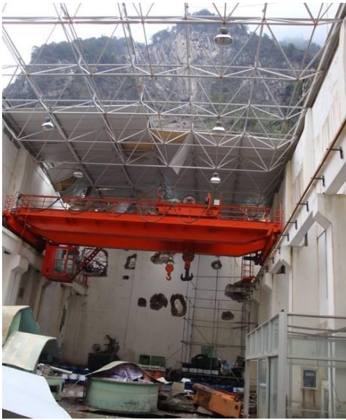
Figure 102: Shapai powerhouse showing damage from ‘evil dancing rock’ impacts (photo from Charlewood et al., 2009).
