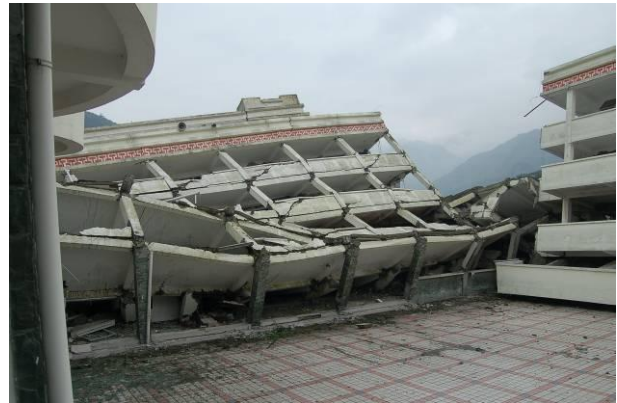
Figure 60: Column Hinging - Classroom Block 1.
