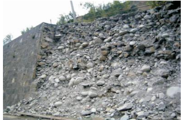
Figure 111: Collapsed section of gravity retaining wall.
