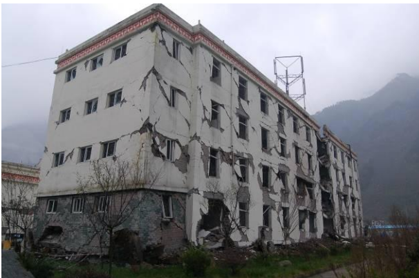
Figure 58: Dormitory Block – partial collapse.
