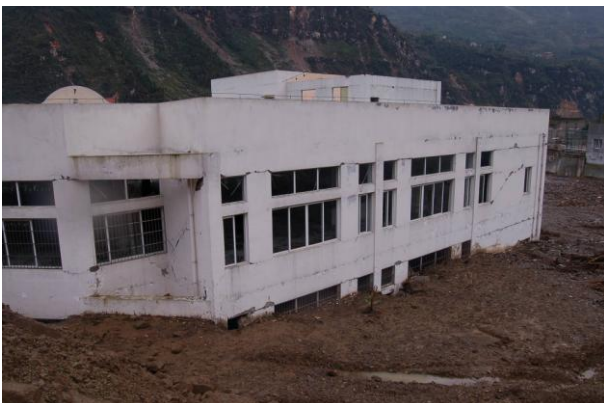
Figure 110: School building partially buried by debris flow in Beichuan.
