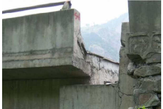
Figure 85: Longitudinal movement at abutment in excess of 600 mm.
