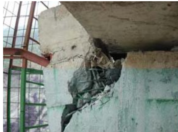
Figure 91: Impact damage of external shear key.
