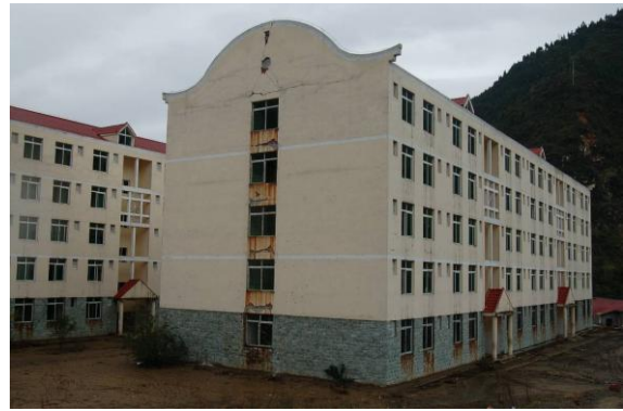
Figure 73: Classroom Block of the school Beichuan, regular structure, minor damage.
