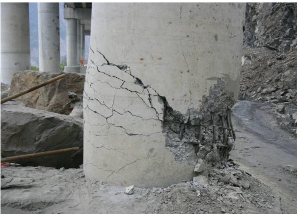
Figure 83: Buckling of main reinforcing bars, spacing of stirrups well in excess of 300 mm.
