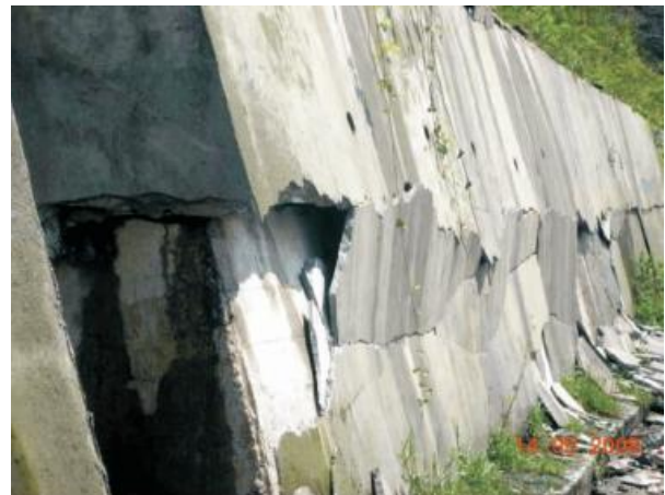
Figure 112: Cracked concrete retaining wall.
