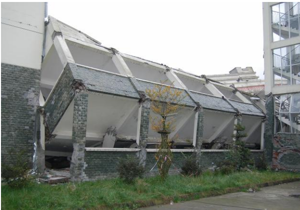
Figure 57: Administration Block – complete collapse.
