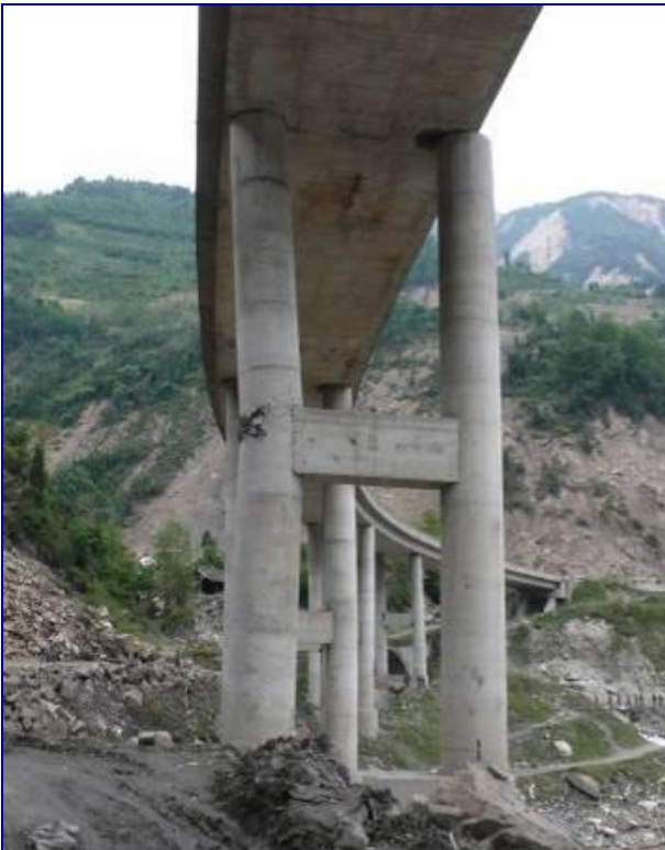
Figure 82: Large lateral displacement (800 mm) of the bridge deck and damage to bridge pier.
