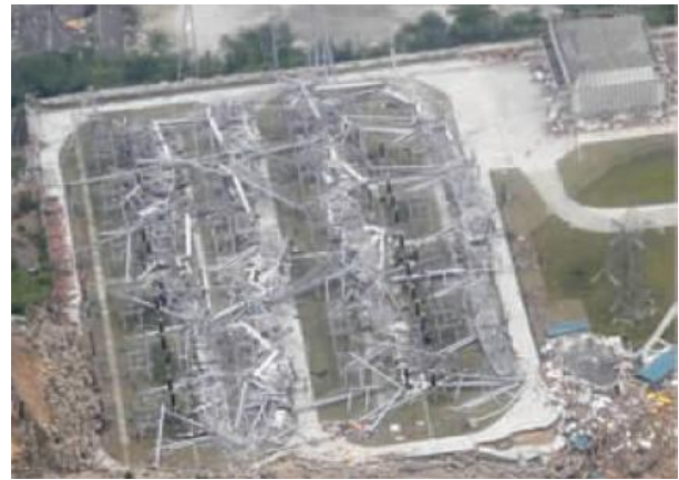
Figure 119: Destruction of substation in earthquake.
