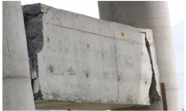
Figure 86: Fracture of main bars in the cross beam, large cracks and ineffective portal action.
