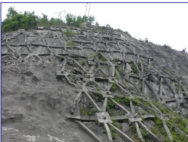
Figure 116: Anchored wall generally performed well.
