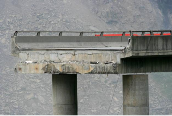
Figure 81: Collapse span end seating – note the lack of restraint bolts and loss of vertical support.
