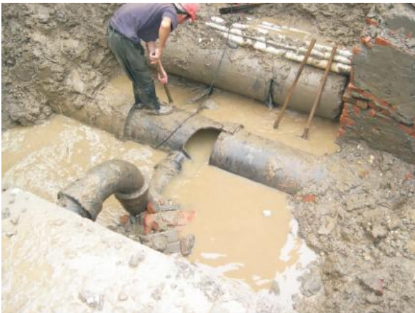
Figure 121: Damage and repair to water supply pipeline.
