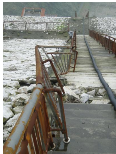
Figure 100: Deformation of Zipingpu dam downstream face reflecting settlement during earthquake.
