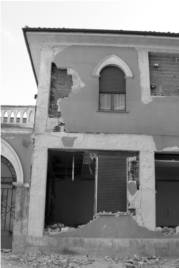
Figure 13: Masonry infill out-of-plane failure (L'Aquila).
