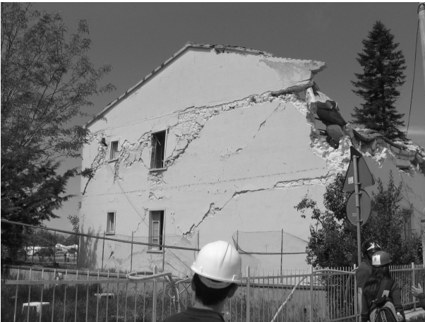
Figure 9: Damage concentration at diaphragm level (Onna).
