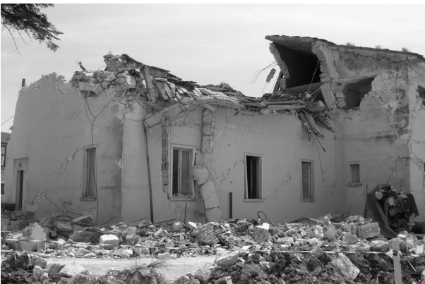
Figure 10: Collapse of walls with R/C ring beam at roof level (Onna).
