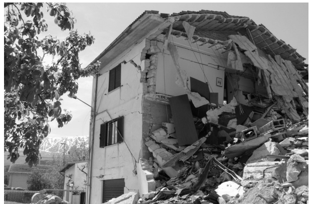
Figure 17: Damage due to deficient performance of perforated masonry diaphragm system (Onna).
