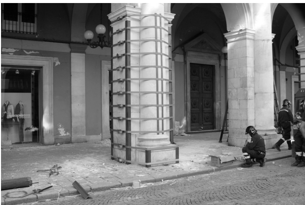
Figure 20: Damaged column stabilized with belts (L'Aquila).
