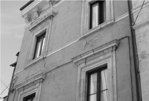
Figure 8: Damage in spandrel (San Gregorio).
