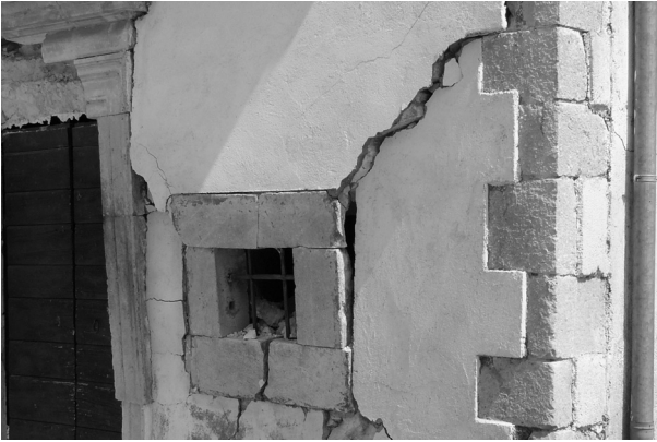
Figure 7: Damage adjacent to openings (San Gregorio).
