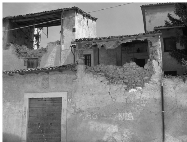
Figure 5: Out-of-plane failure of walls (San Gregorio).
