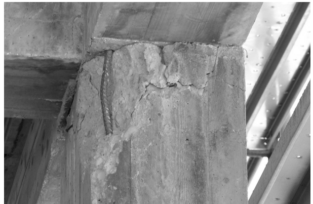
Figure 18: Plastic hinging and reinforcement buckling at the top of a column (Onna).
