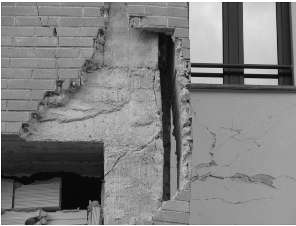
Figure 12: Veneer out-of-plane failure (L'Aquila).
