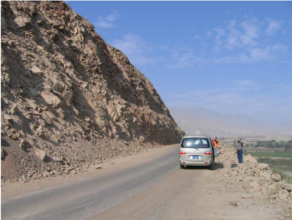
Figure 18. Rock slide above road in Andes foothill
