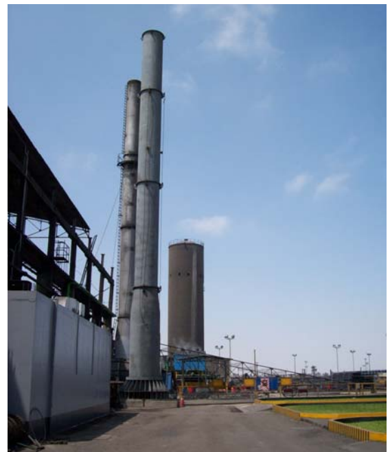
f). Exhaust fume stacks
