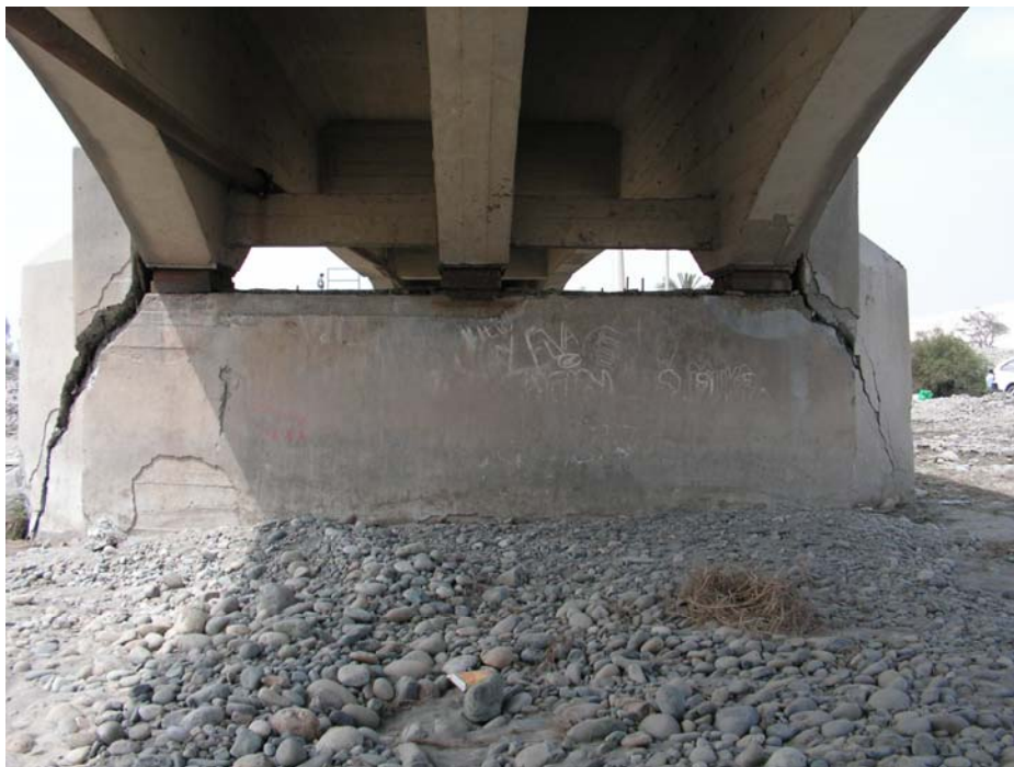
Figure 106. Damage to restraining walls
