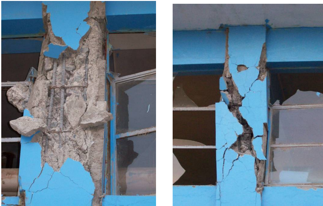
Figure 89. Short Column Failure - Ica Regional Hospital
