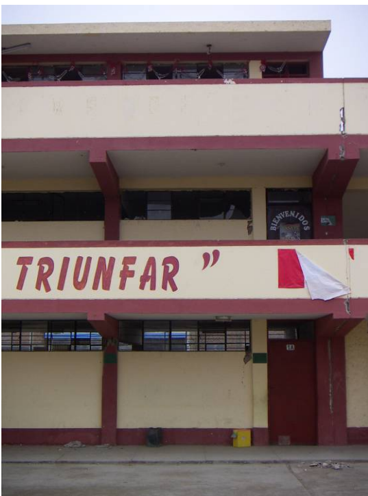
Figure 77. Damaged School - Canete
