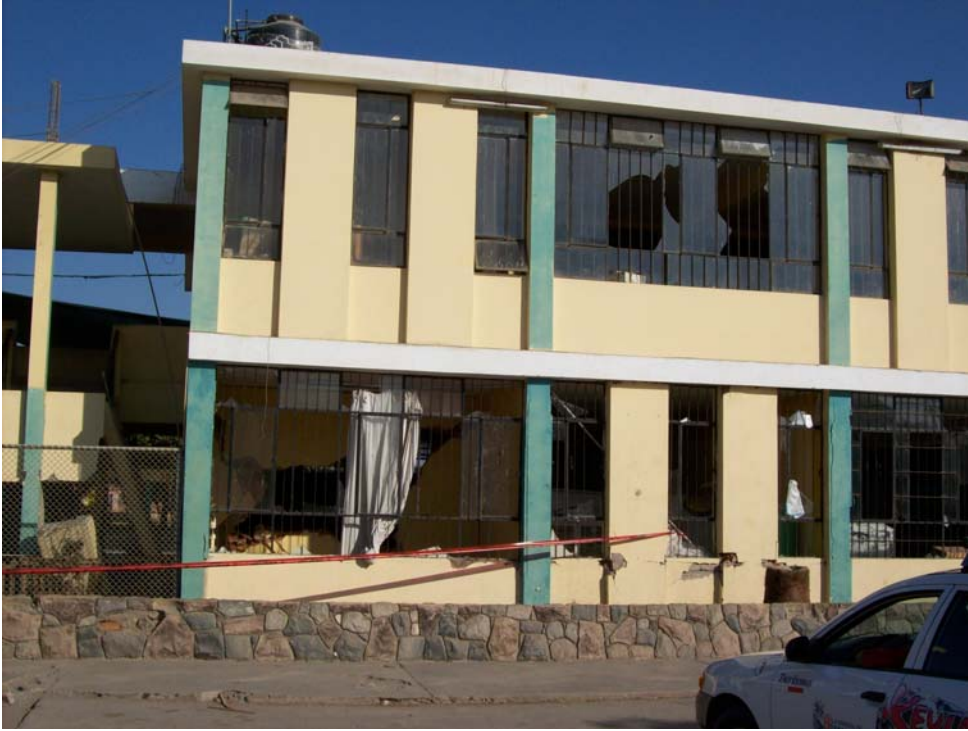
Figure 84. Glass damage at an Ica school
