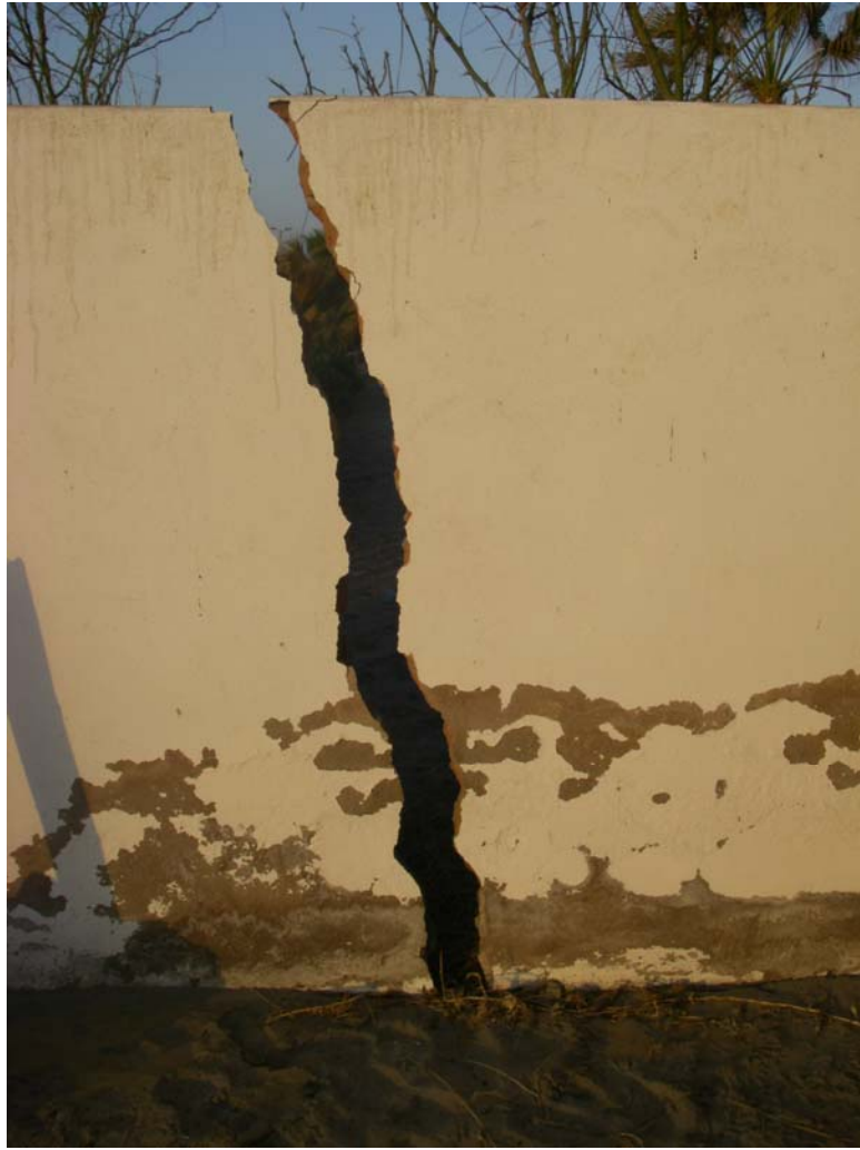
Figure 28. Liquefaction-induced offset to wall in Paracas
