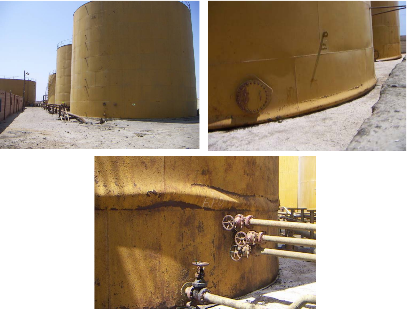
Figure 101. Tank Damage - Blue Pacific Oil
