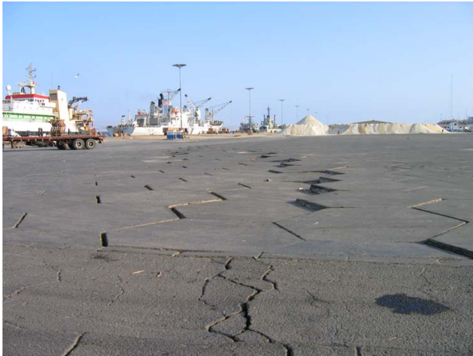
Figure 112. Settlement of backfilled areas behind wharf
