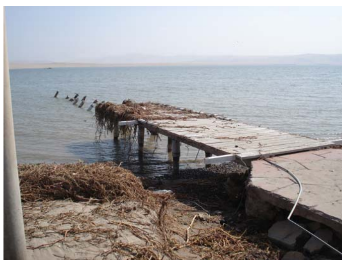
Figure 108. Tsunami damage to pier on Paracas coast Photo courtesy Alfonso Rey
