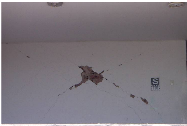
Figure 65. Diagonal cracking of infill masonry panel
