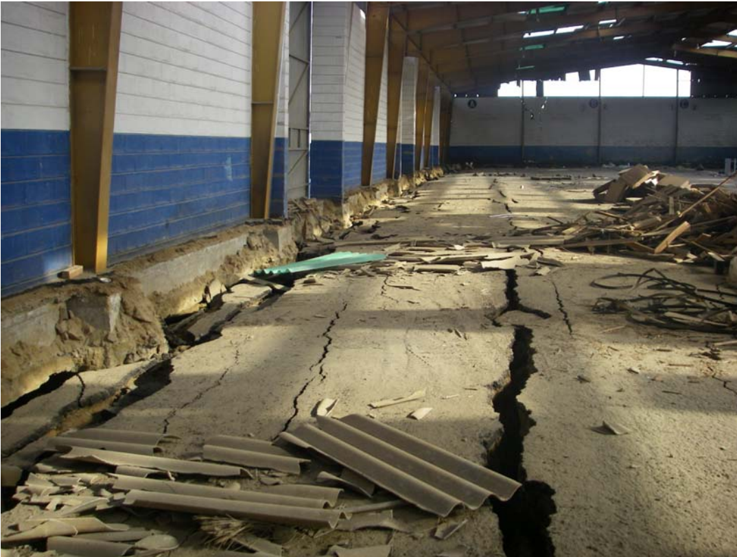
Figure 29. Ground subsidence in wharf shed at Port San Martin
