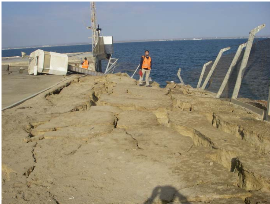
Figure 110. Wharf damage - Port San Martin
