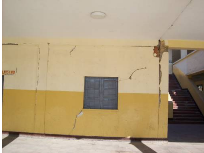
Figure 81. Infill wall damage - Ica
