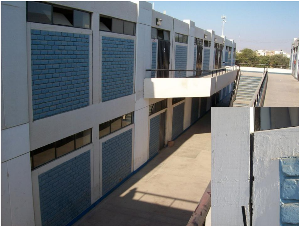
Figure 85. Spandrel separation at an Ica school
