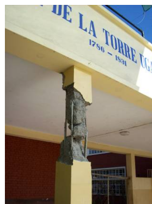
Figure 80. Column Damage - Ica
