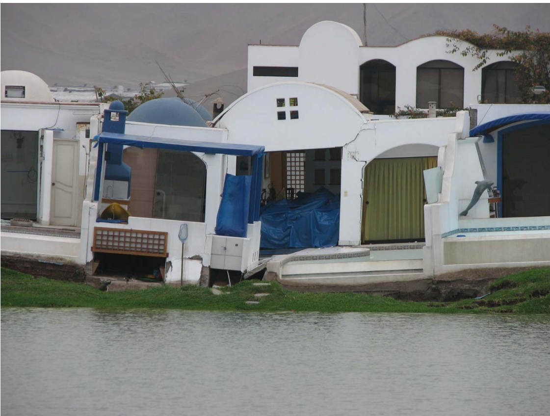
Figure 30. Liquefaction damage at Las Lagunas Photo courtesy Alfonso Rey
