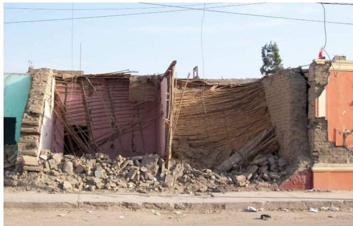
Figure 56. Typical Adobe House Damage
