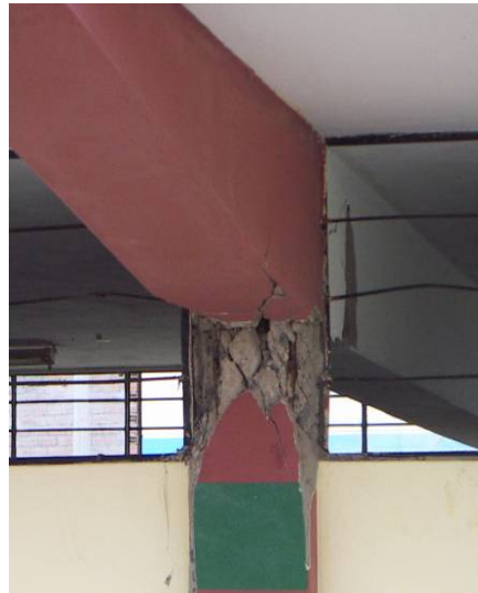
Figure 78. Column Damage - Canete
