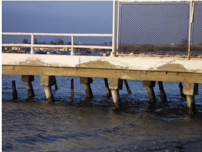
Figure 109. Structural damage to pier Photo courtesy Alfonso Rey
