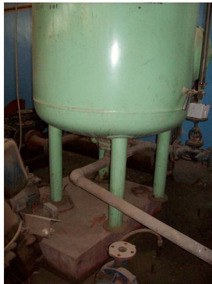
Figure 91. Unsecured Building Plant - Ica Regional Hospital
