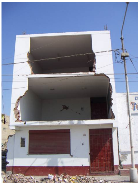
Figure 64. Pisco Confined Masonry Buildings with panel damage
