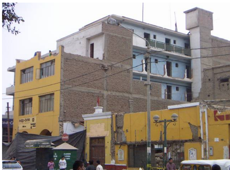
Figure 66. Brick panel damage - Ica
