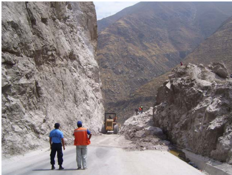
Figure 19. Failure of cut slope Photo – Ministry of Transport and Communications
