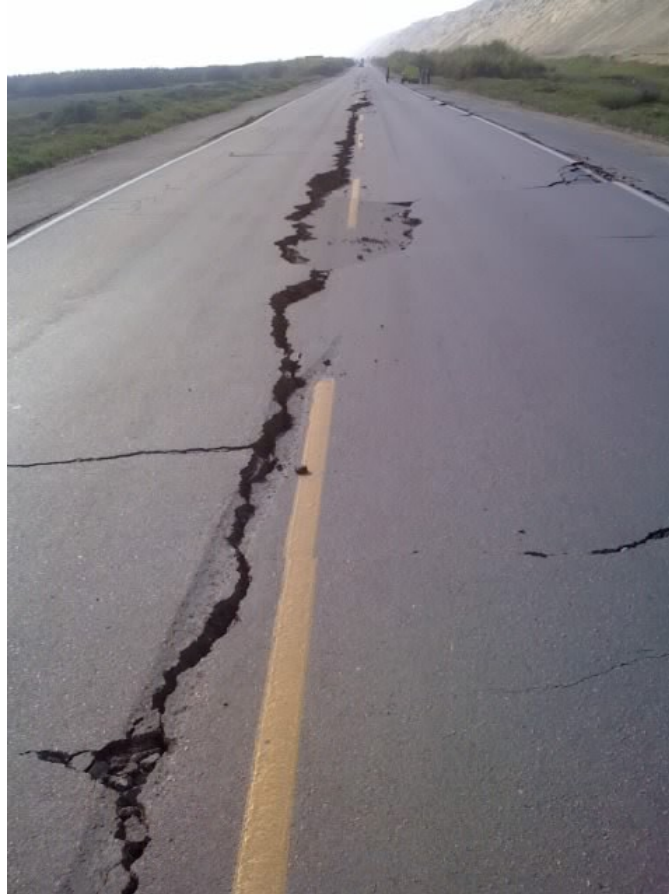
Figure 22. Low embankment failure Photo – Ministry of Transport and Communications
