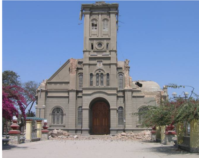
Figure 55. Collapsed church roof - Ica
