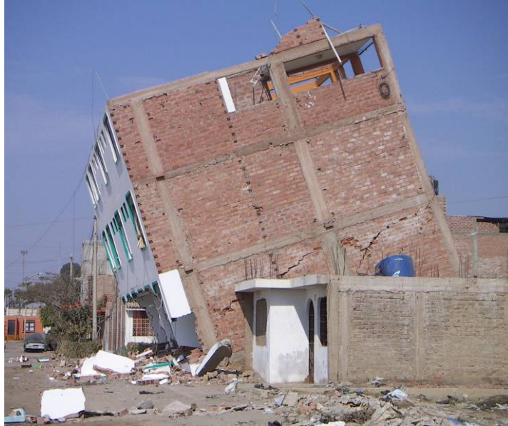
Figure 67. First Floor Collapse - Pisco Residential Buildings
