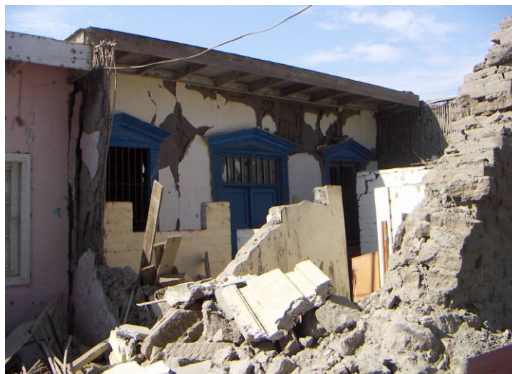
Figure 57. Collapsed Adobe House - Pisco
