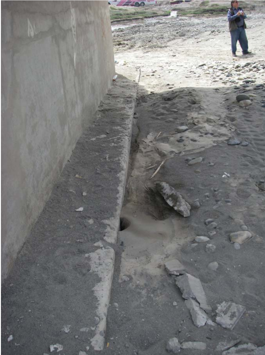
Figure 27. Ejecta around bridge abutments
