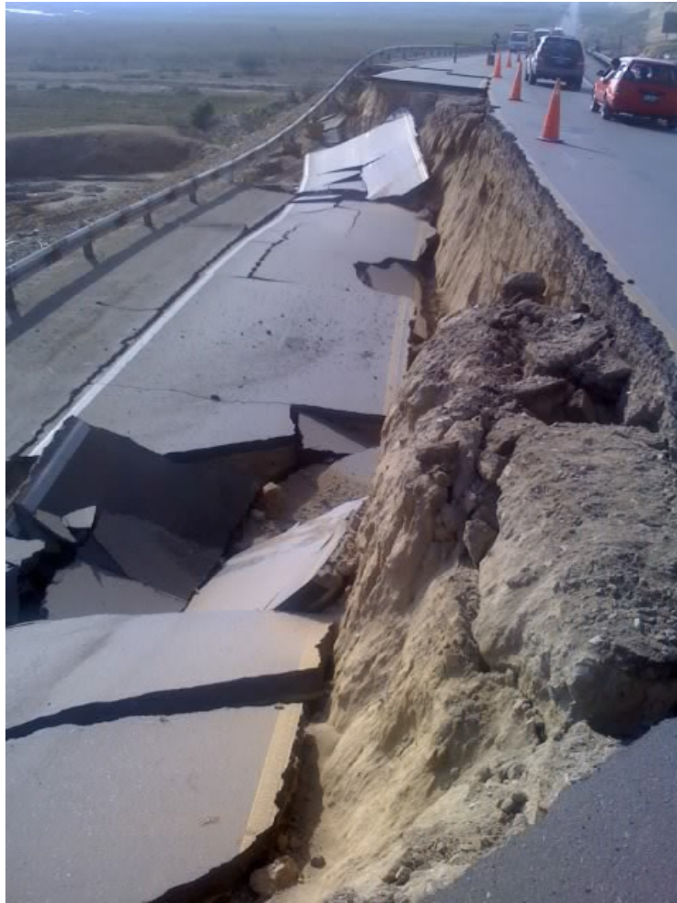
Figure 24. Larger slip on Pan American Highway Photo – Ministry of Transport and Communications
