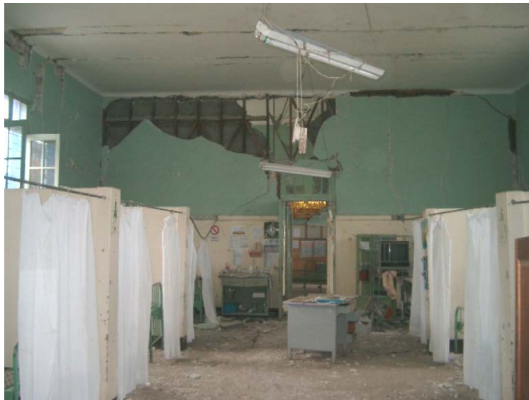
Figure 13. Damage to hospital treatment room in Ica Regional Hospital
