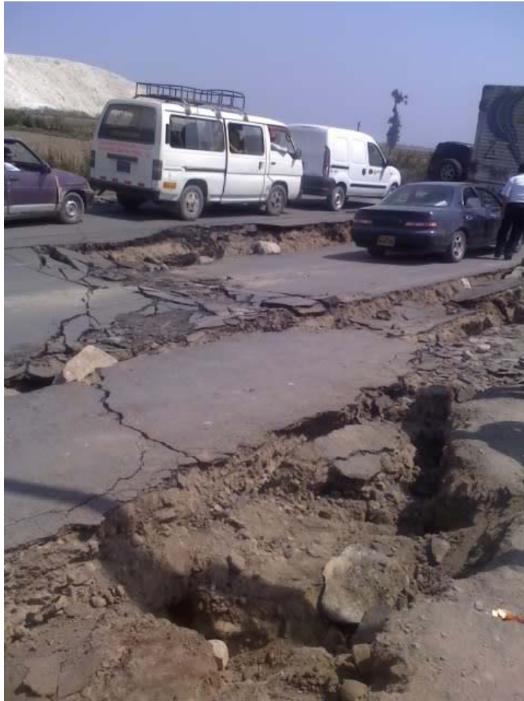
Figure 23. Damage to the Huamani Bridge southern embankment Photo – Ministry of Transport and Communications
