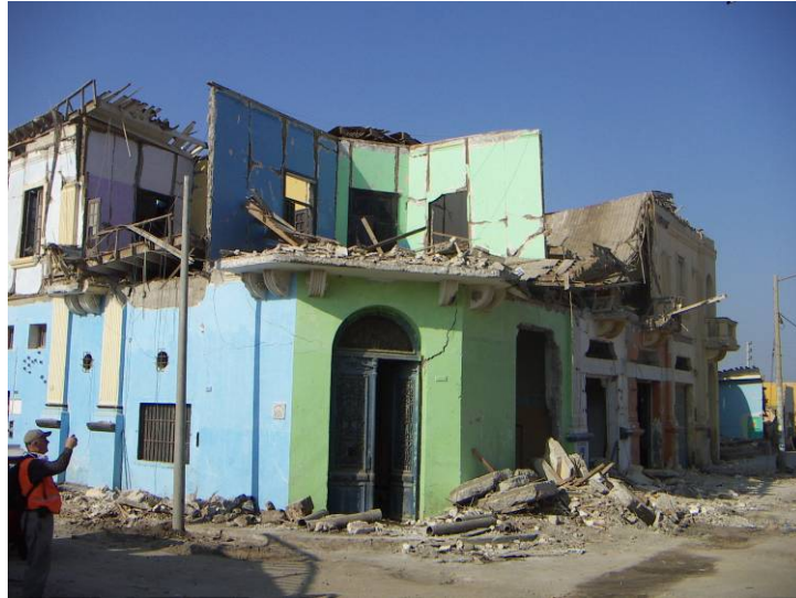
Figure 58. Damaged Two Storey Adobe Buildings - Pisco
