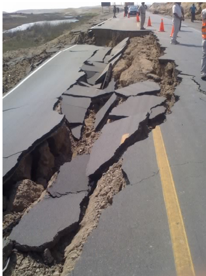
Figure 21. Typical embankment failure as a result of liquefaction Photo – Ministry of Transport and Communications
