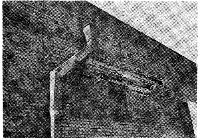
FIG. 3 - Loss of outer wites of bricks
