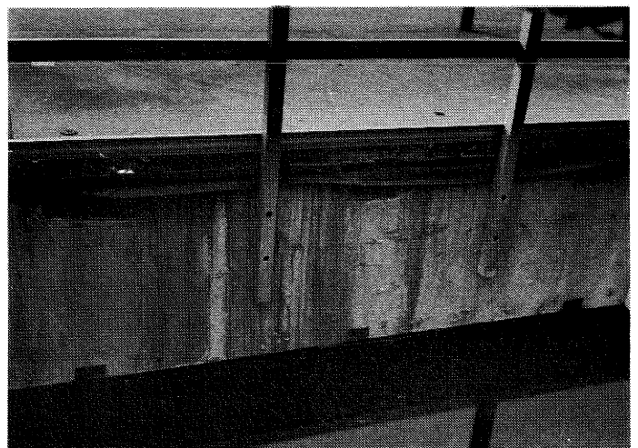
FIG. 7 - Position from which panel fell, killing student. Railing added after accident.
