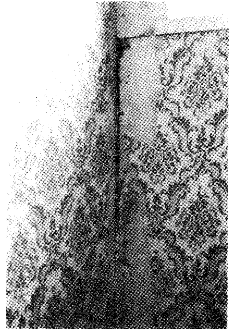
Figure 4.1.4 : Typical damage to joints between sheets of wall linings
