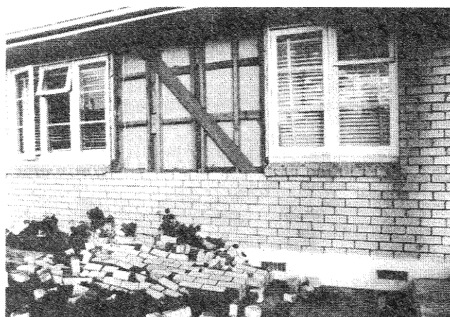
Fig. 4.1.14 : A collapsed panel of brick veneer
