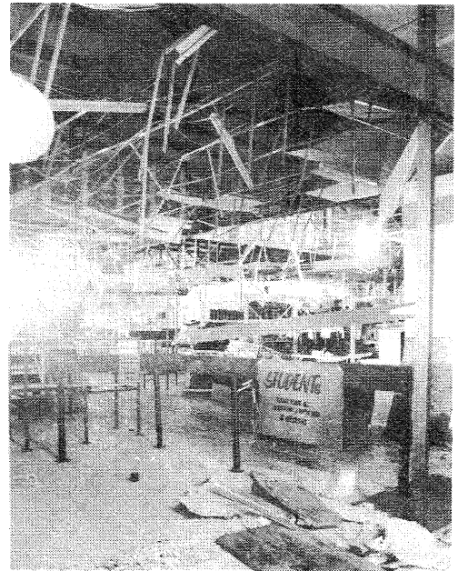
Figure 4.2.1 : Riverslea Shopping Centre suspended ceiling collapse
