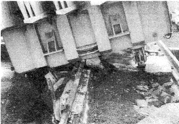
Fig. 7.1.3 : Close up view. Note twisted holding down bracket
