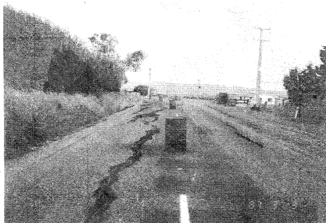
Fig. 3.8 : Cracking in Thompson Rd. which, at this location, is on the crest of the stopbank along the Rangitaiki River
