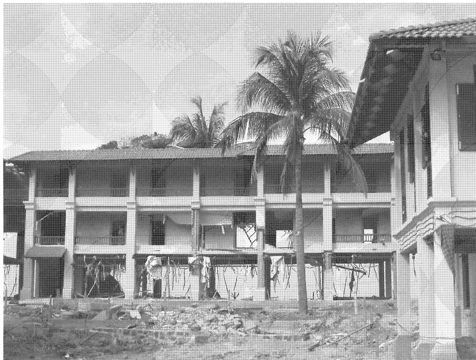
Figure 13. One of resorts at Khao Lak located a few hundred metres from the shoreline, where the highest tsunami run-up (12m) occurred. Water entered rooms even on the third floor, and in-fill block walls and windows on the first and second floors were punched out (Photo ED).
