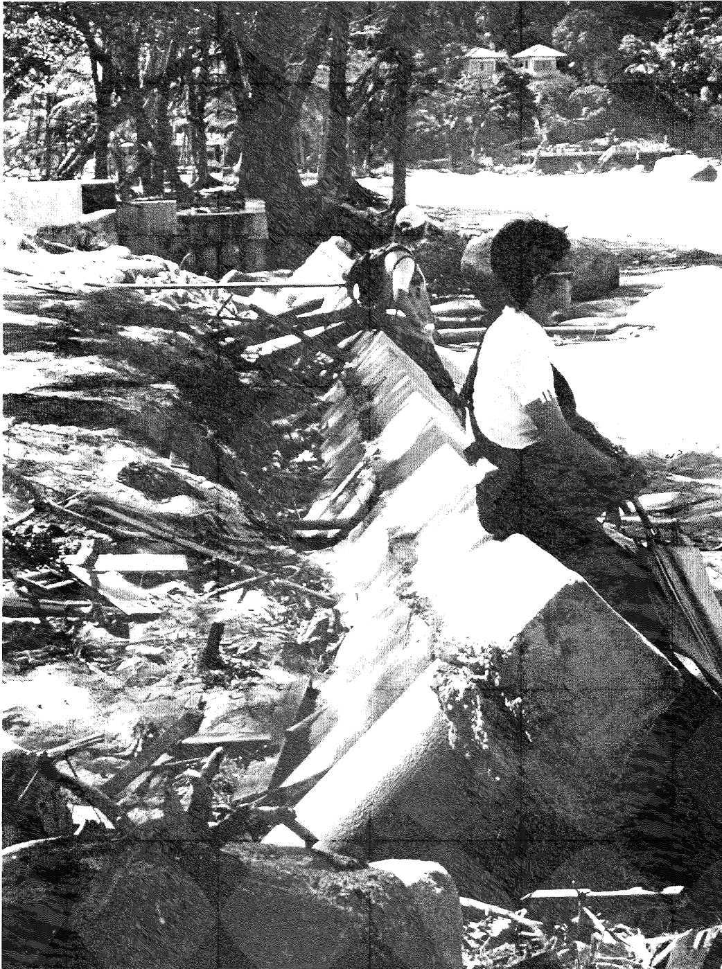
Figure 18. Receding waters (out-rush) caused collapse of most seawall defences from behind due to scouring (Photo RB).
