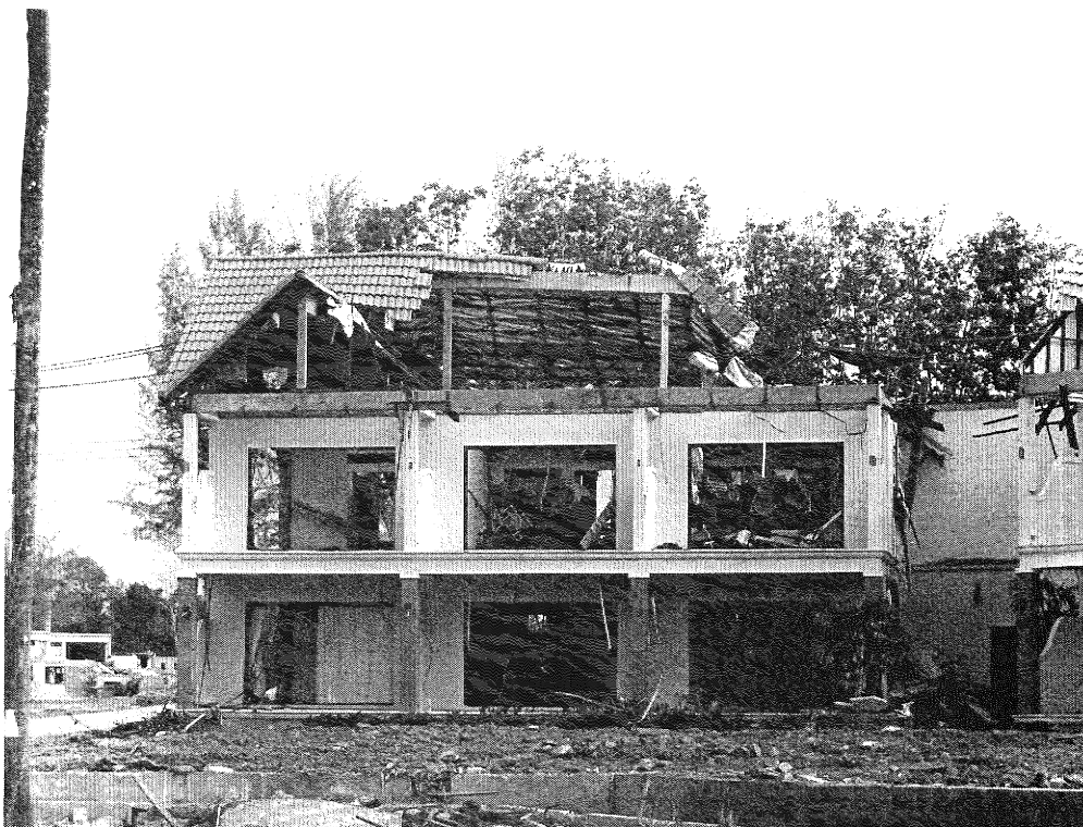
Figure 5. Missing roof tiles indicate the tsunami torrent depth exceeded nine metres at this location in Khao Lak (Photo ED).
