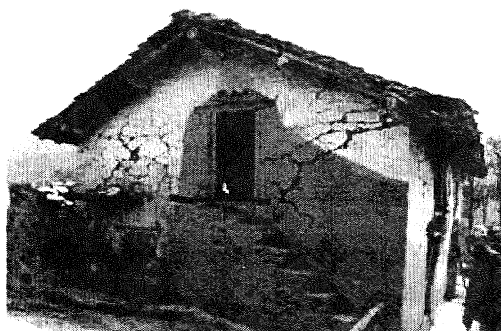
Figure 5: Shear cracking of wall piers.
