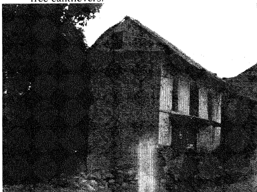
Figure 3: Shear and vertical cracking
