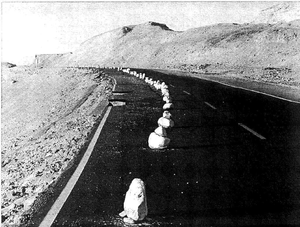
Figure 8. Damage to the Pan American highway from failure of the slopes beneath the highway. Damage like this was widespread on the highways along the 300km long earthquake rupture zone, creating some considerable traffic hazards.
