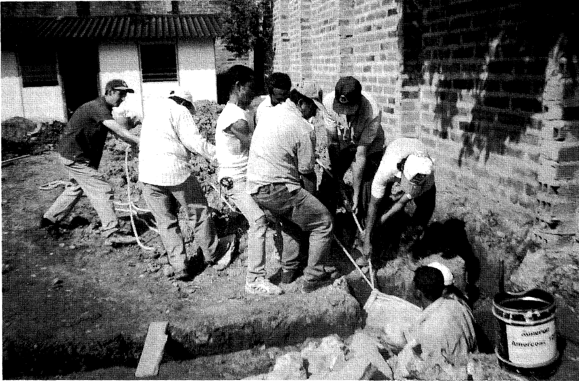
Figure 5. A construction gang removes a large boulder from an excavation into rubble debris-flow deposits ( Q_{fm} ) near accelerograph station POL.
