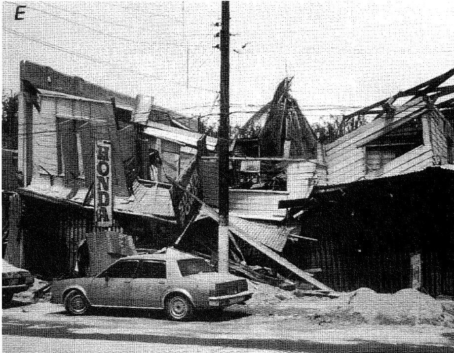
Figure 5: Building damage by roof collapse due to ash-loading (after [30]).
